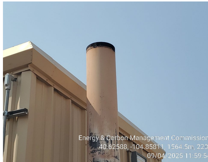
West separator burner stack
