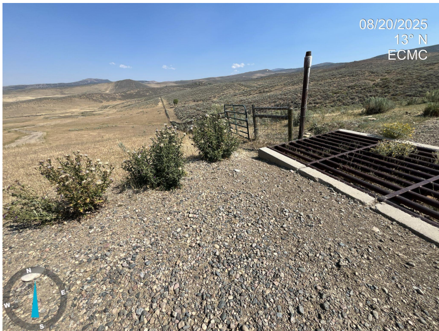
Photo 7. Photos 7-8 taken at the entrance of the access road. The cattle guard and gate remain present. Weeds, such as Bull thistle observed along the access road.
