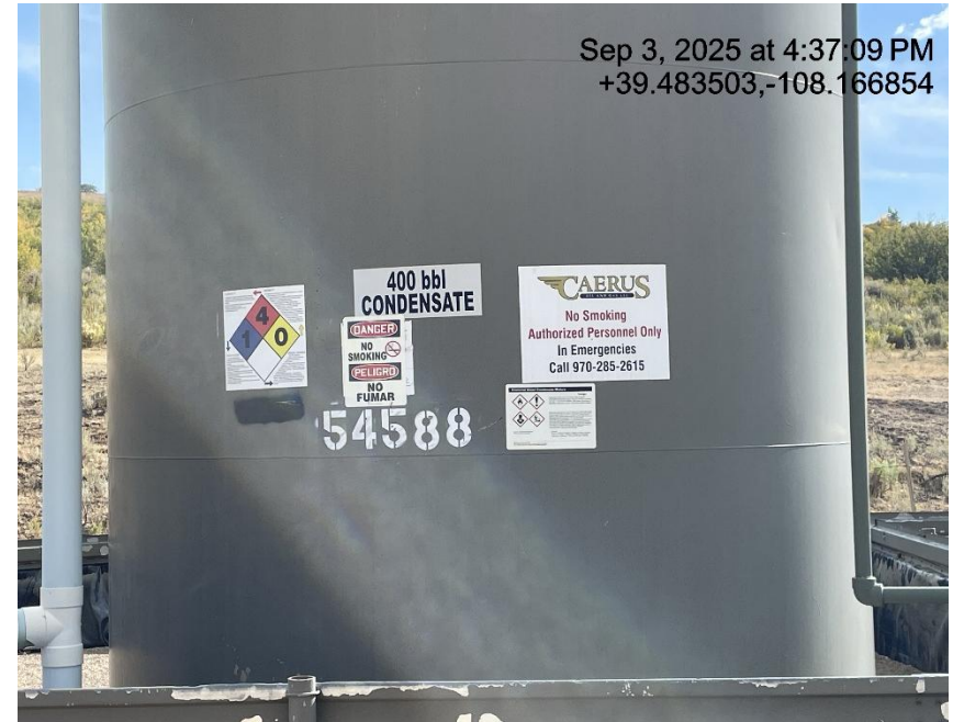
Photo # 6290 Tank label has previous operators name/not in compliance with CECMC Rule 605
