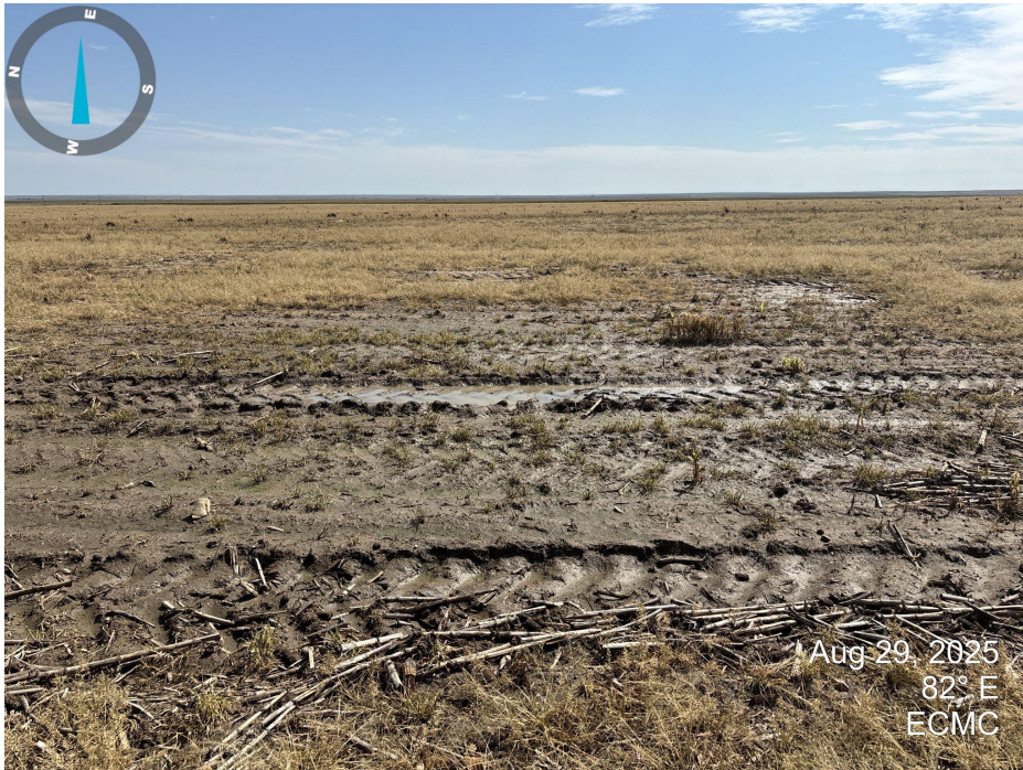
Photo 7. Picture taken approximately at the northwest side of the evap pond looking east across a low spot. This area appears to have some subsidence and water pooling.
