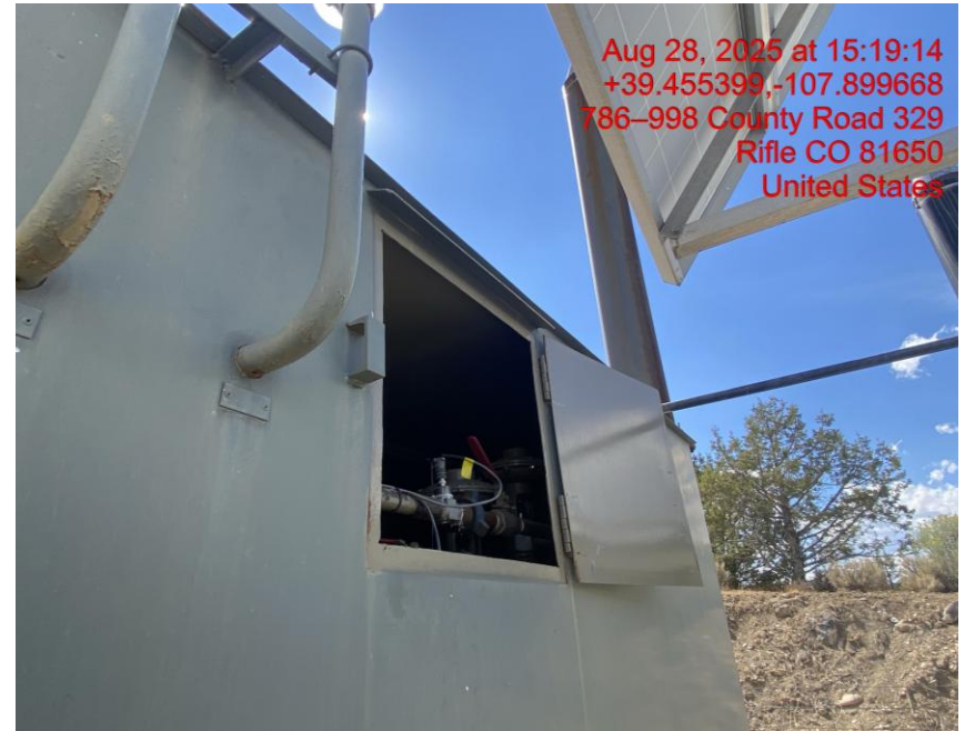
Wildlife Entry Hazard – Photo #00519
