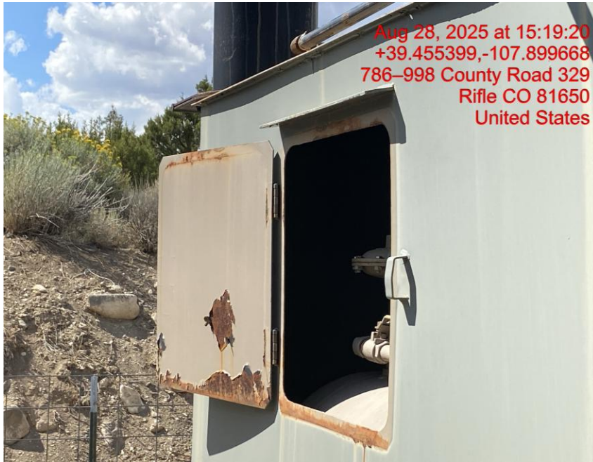
Wildlife Entry Hazard – Photo #00520
