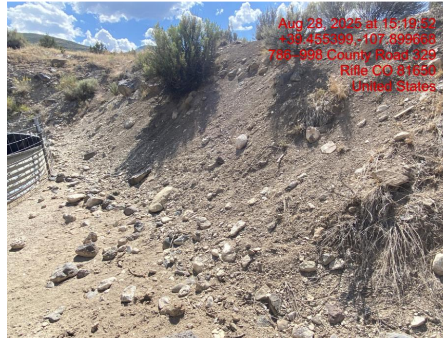
Insufficient Erosion Controls – Photo #00521
