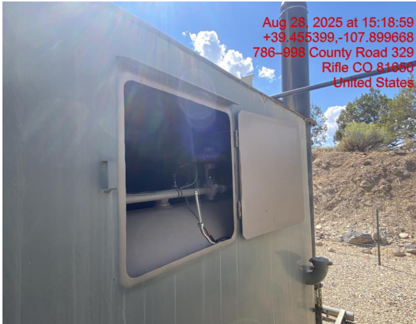
Wildlife Entry Hazard – Photo #00518
