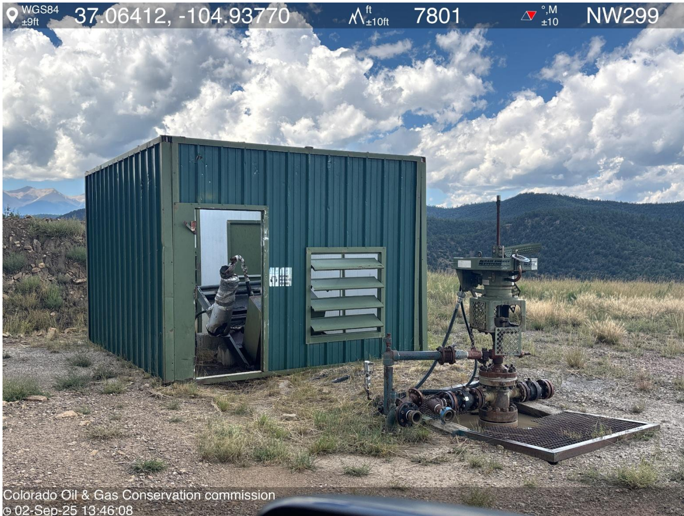
PHOTO 3: WELLHEAD AND EQUIPMENT.
