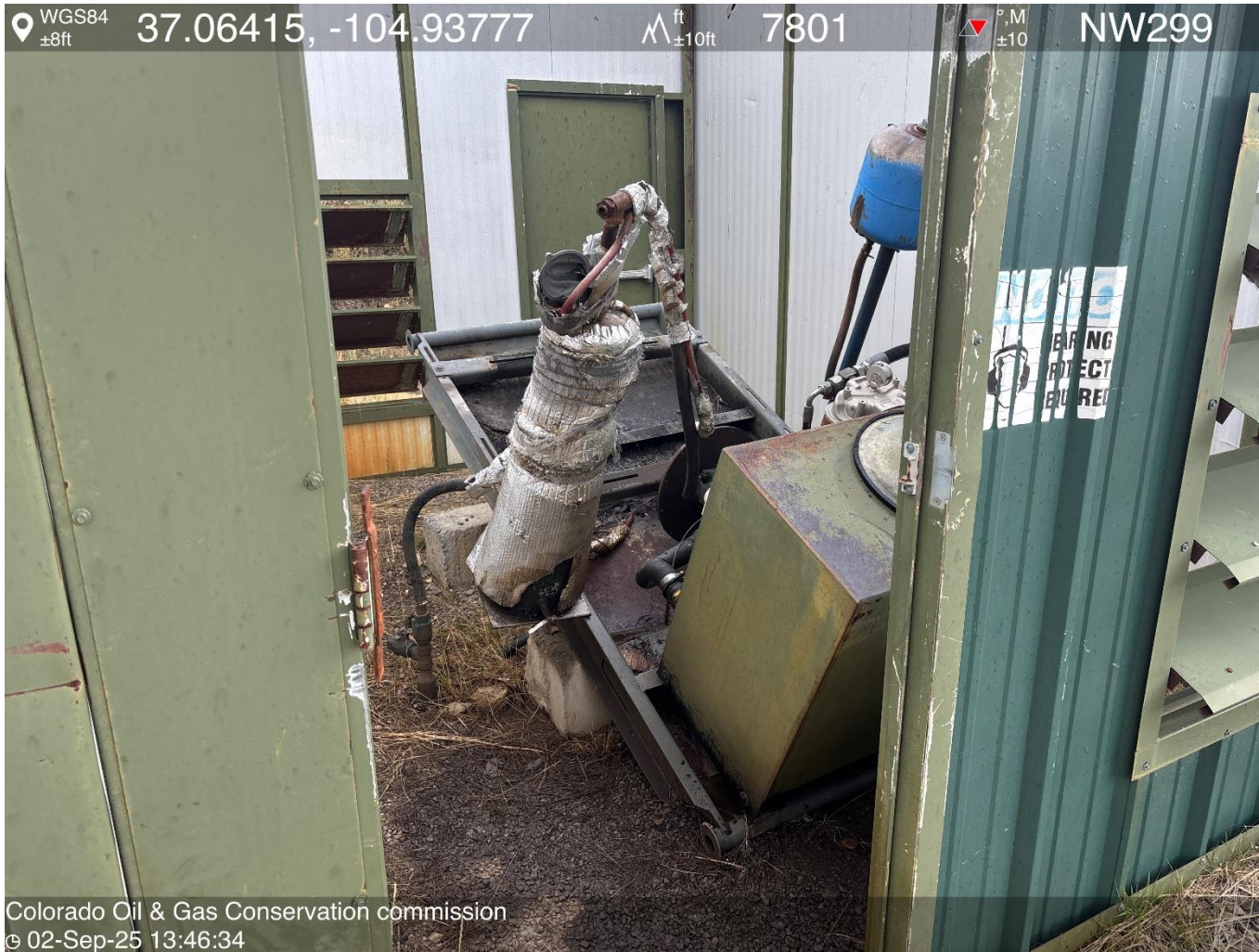
PHOTO 4: UNUSED EQUIPMENT (PRIME MOVER ENGINE SKID SOUND WALLS). REMOVE UNUSED EQUIPMENT PER RULE 606. CA DATE 10/3/2025.
