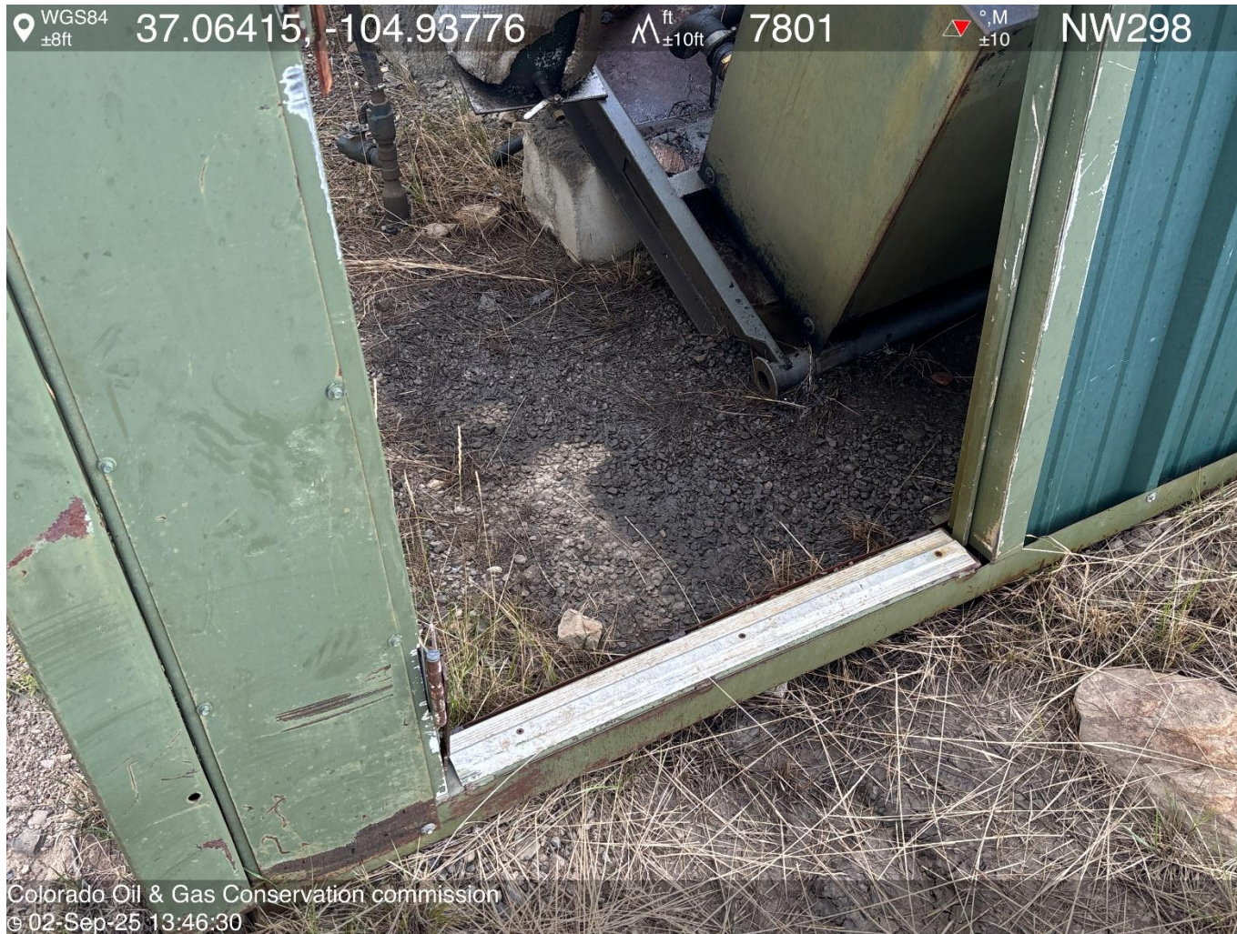
PHOTO 6: Impacted soil identified at various locations through out location. Conduct maintenance on equipment, cleanup stained material and review self inspection processes. COMPLY WITH RULE 1002,.(2).D. CA DATE 9/9/2025.
