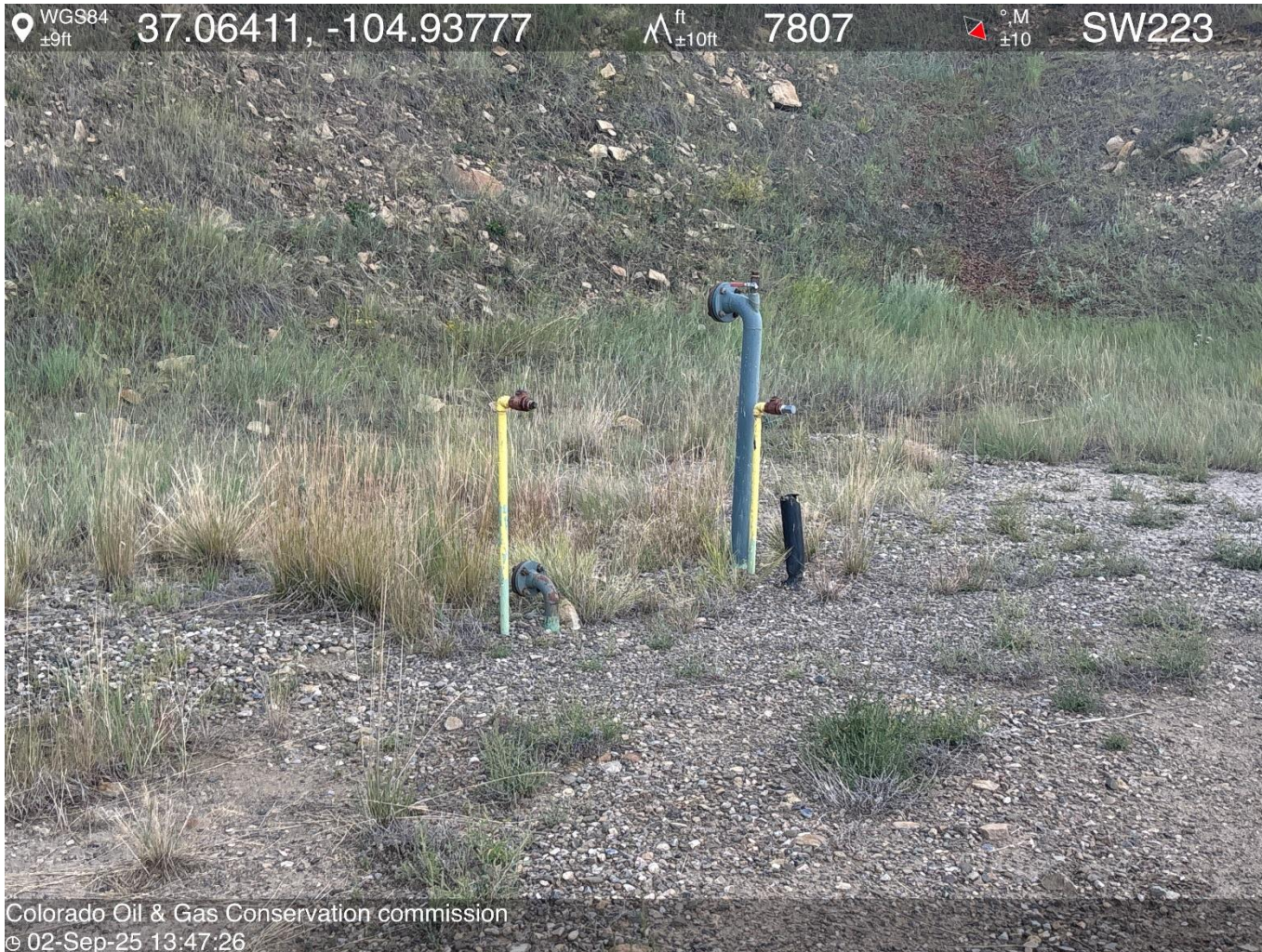
PHOTO 5: UNUSED EQUIPMENT (2- 1" RISERS AND 2-2" RISERS). REMOVE UNUSED EQUIPMENT PER RULE 606. OR MARK RISER WITH A PERMANENT MARKING. CA DATE 10/3/2025.
