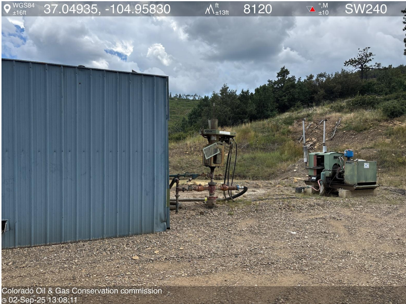
PHOTO 3: WELLHEAD AND EQUIPMENT.
