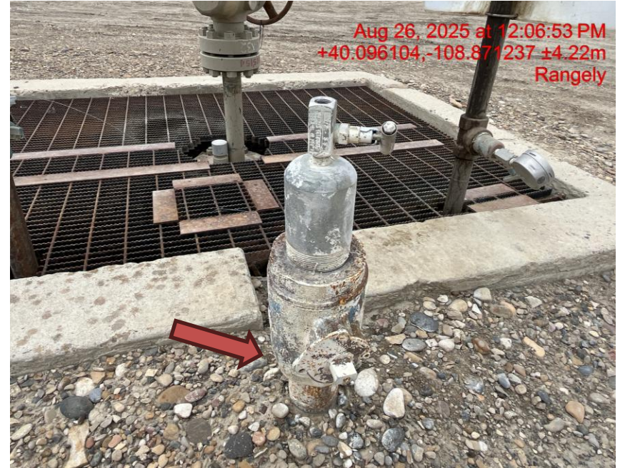
Photo # 2603 Unused flowline lacks lockout tagout (OOSLAT)
