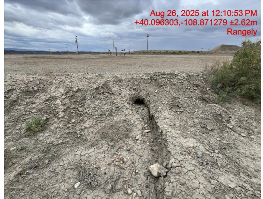
Photo # 2608 Berm needs maintenance
