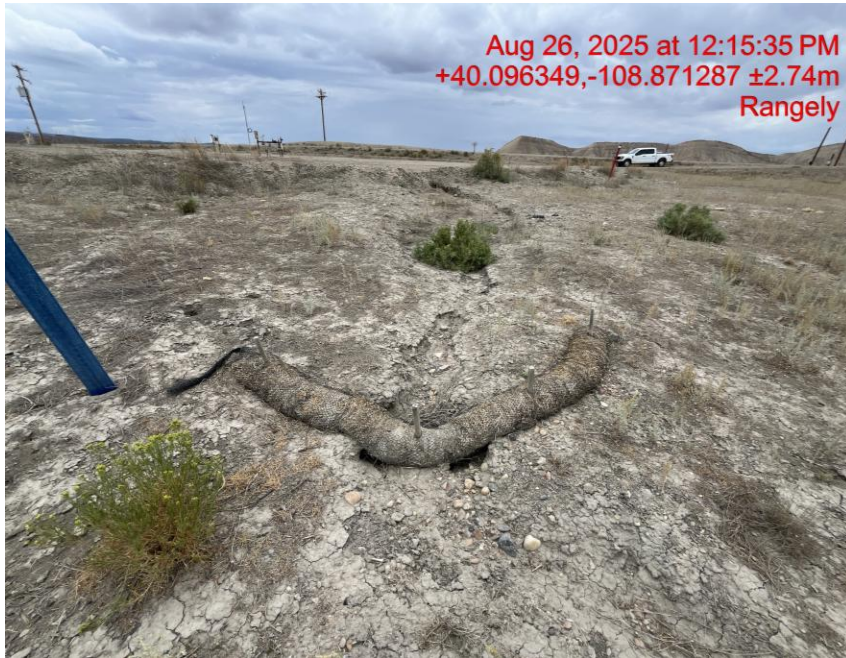
Photo # 2612 Wattles need maintenance
