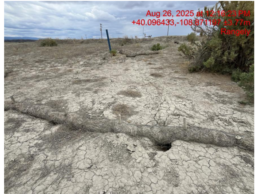
Photo # 2613 Wattles need maintenance
