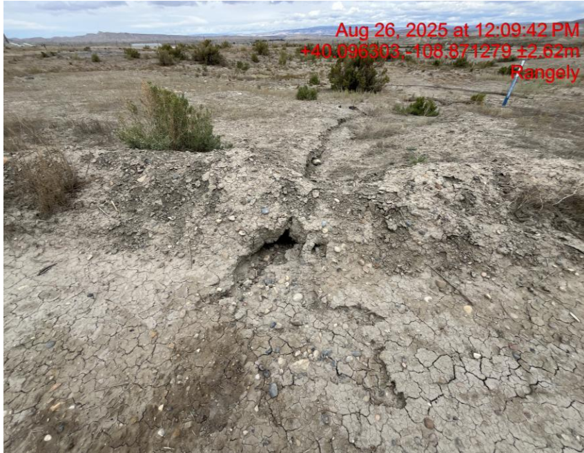
Photo # 2605 Berm needs maintenance
