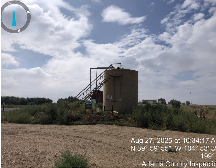
Photo #1 Tanks & weeds.
