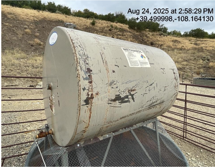
Photo # 3380 Methanol tank lacks required labeling
