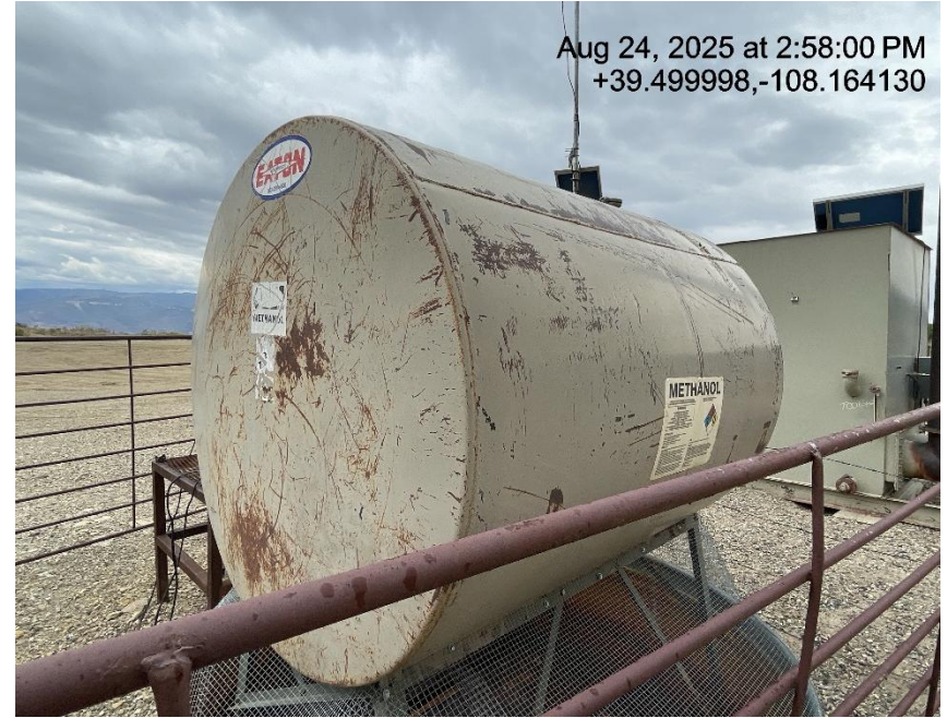
Photo # 3381 Methanol tank lacks required labeling
