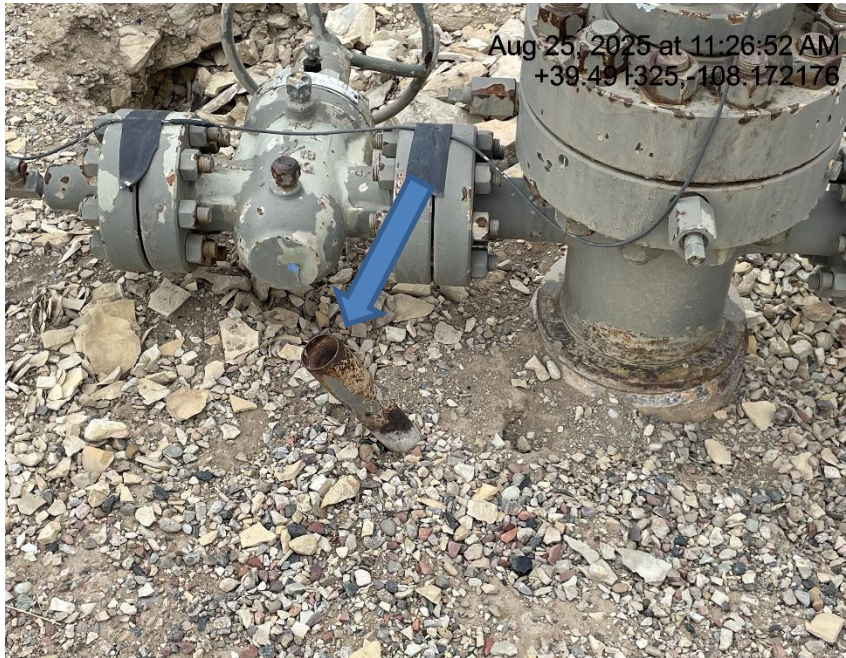
Photo # 3530 Open ended piping near wellhead/wildlife hazard
