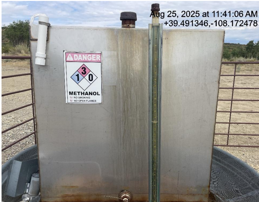
Photo # 3536 Methanol tank lacks required labeling
