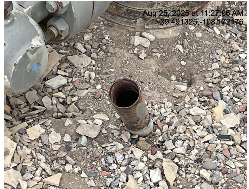
Photo # 3531 Open ended piping near wellhead/wildlife hazard
