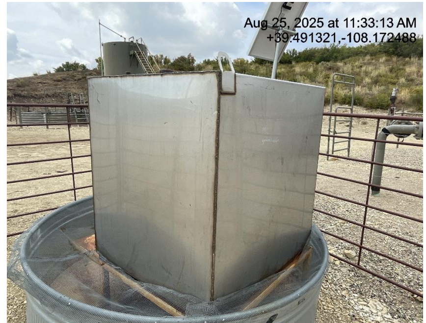
Photo # 3535 Methanol tank lacks required labeling
