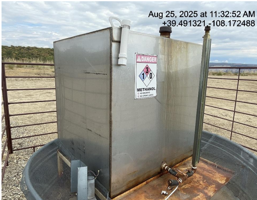
Photo # 3534 Methanol tank lacks required labeling
