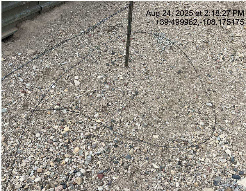
Photo # 3189 Barbed wire fence needs maintenance/wildlife hazard
