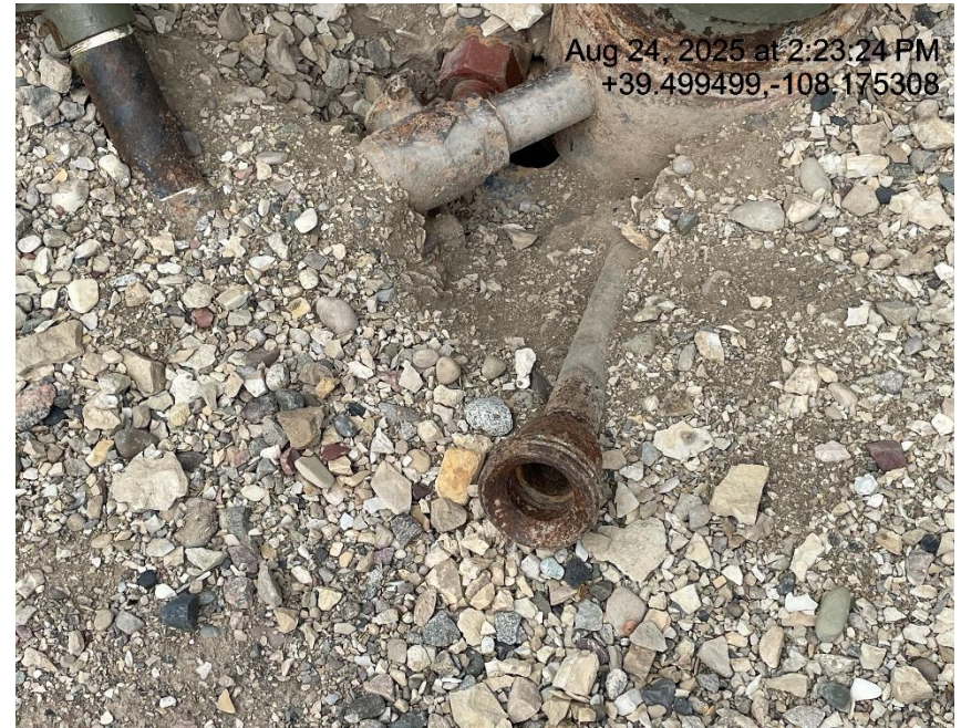
Photo # 3186 Open ended piping near wellhead/wildlife hazard
