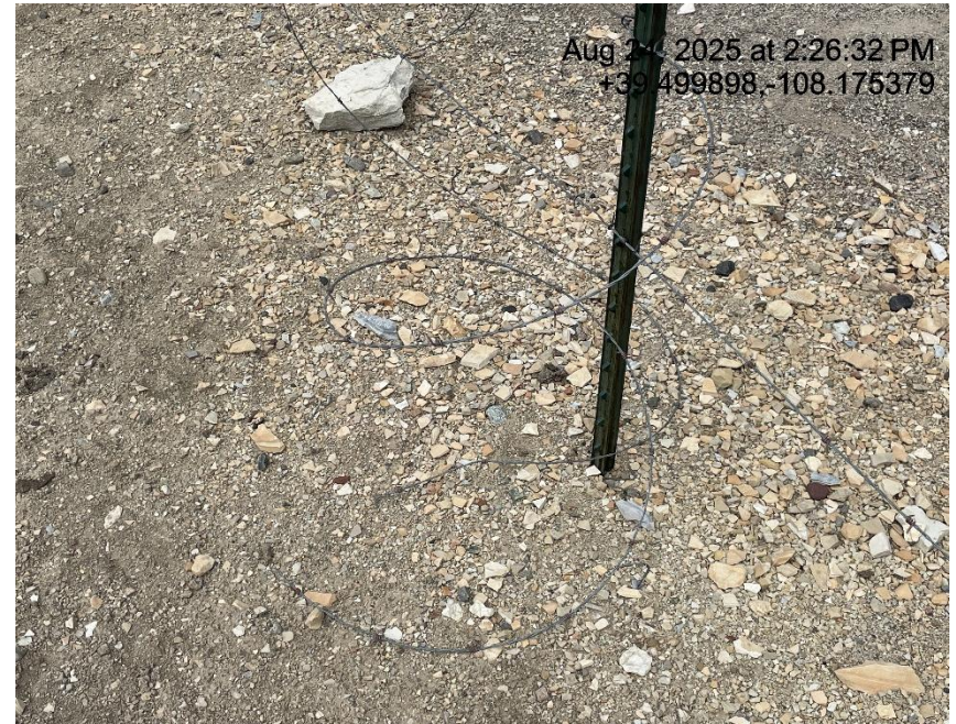
Photo # 3190 Barbed wire fence needs maintenance/wildlife hazard
