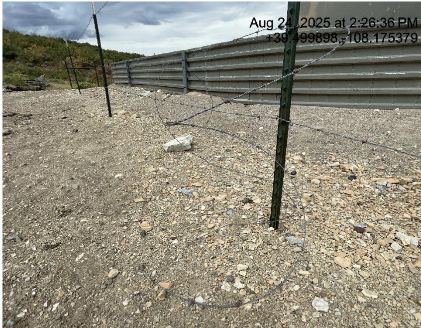
Photo # 3191 Barbed wire fence needs maintenance/wildlife hazard
