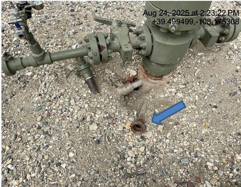
Photo # 3185 Open ended piping near wellhead/wildlife hazard
