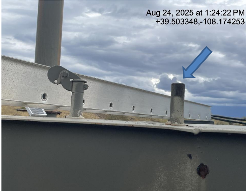
Photo # 3013 Rupture disc vent line does not comply with CECMC pressure safety device rules
