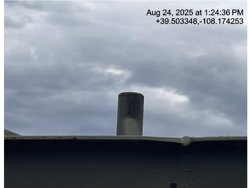
Photo # 3014 Rupture disc vent line does not comply with CECMC pressure safety device rules
