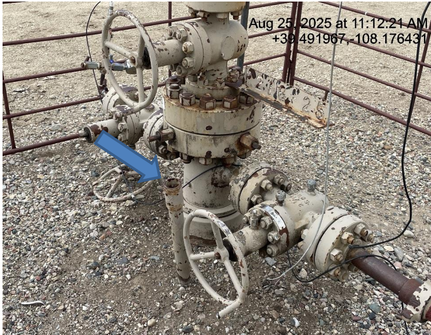
Photo # 3464 Open ended piping near wellhead/wildlife hazard
