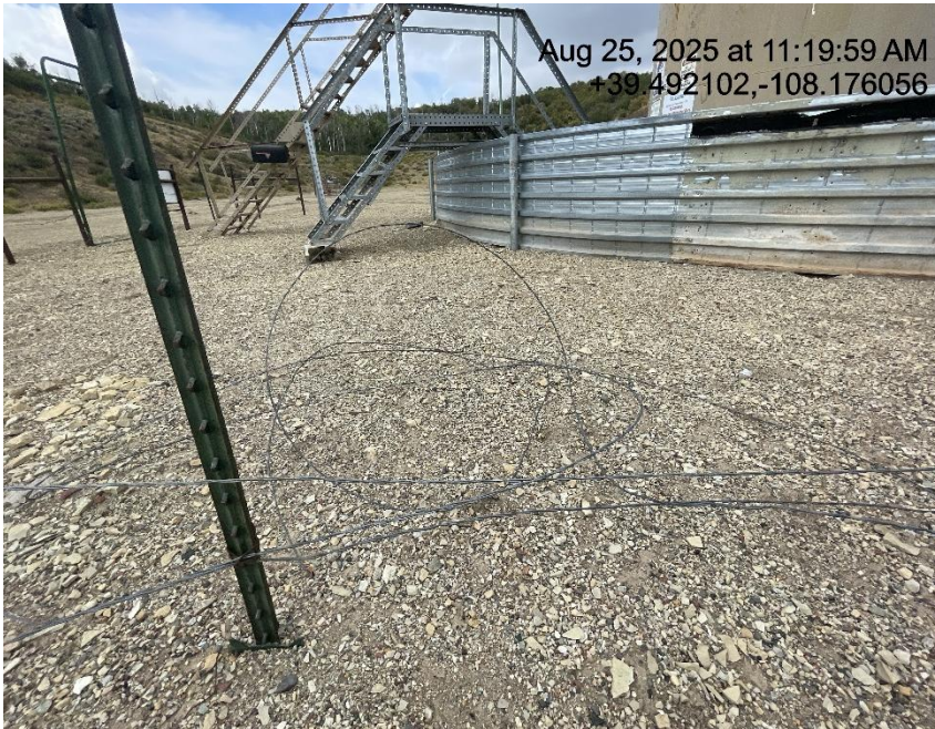
Photo # 3460 Fencing needs maintenance/wildlife hazard
