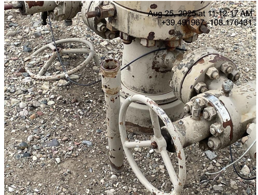
Photo # 3465 Open ended piping near wellhead/wildlife hazard
