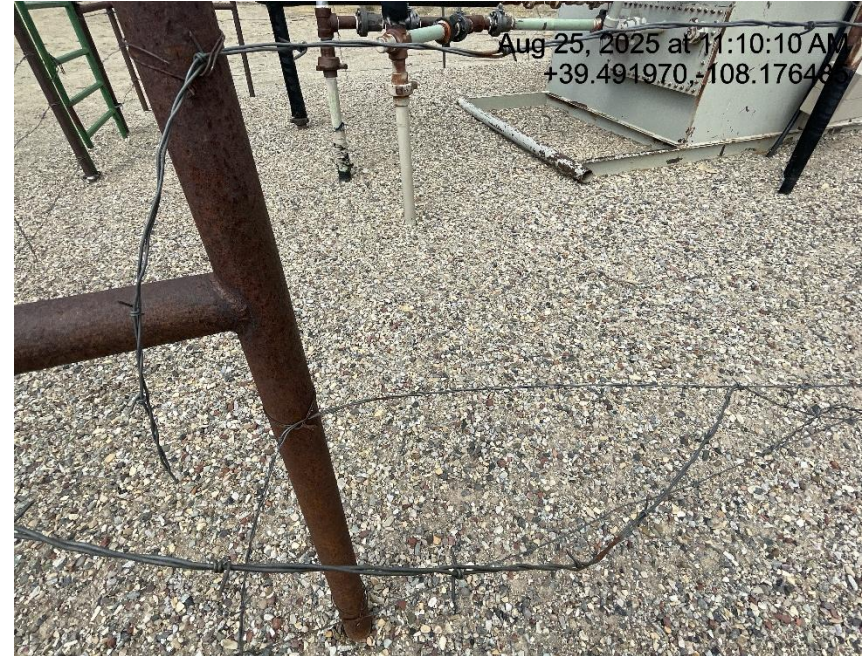
Photo # 3457 Fencing needs maintenance/wildlife hazard
