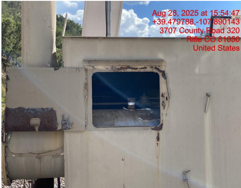
Wildlife Entry Hazard – Photo #00532
