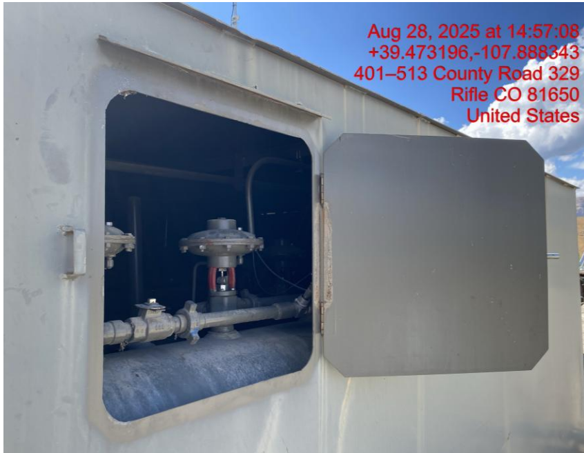
Wildlife Entry Hazard – Photo #00505
