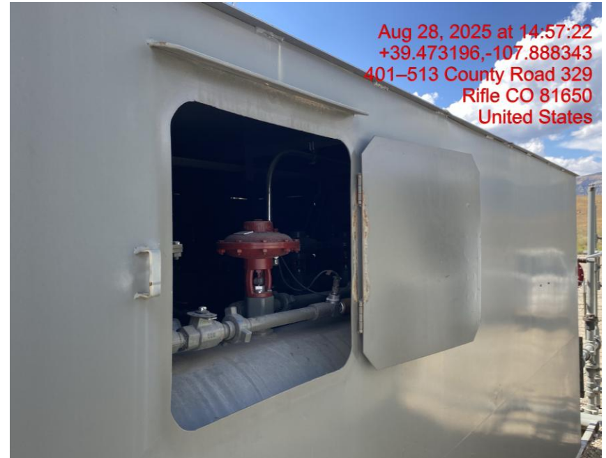
Wildlife Entry Hazard – Photo #00506
