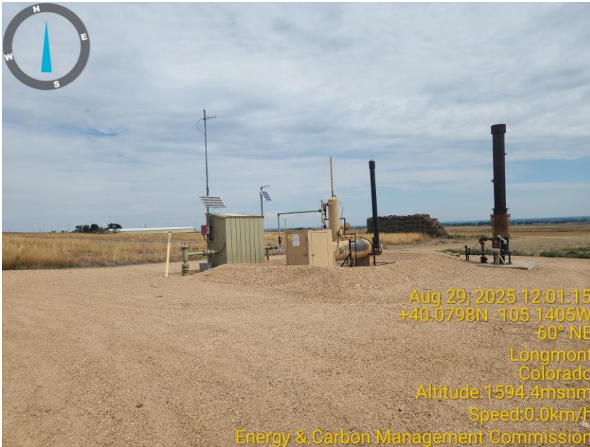
Photo 5 ECD Horizontal Heated Separator & Gas meter run.
