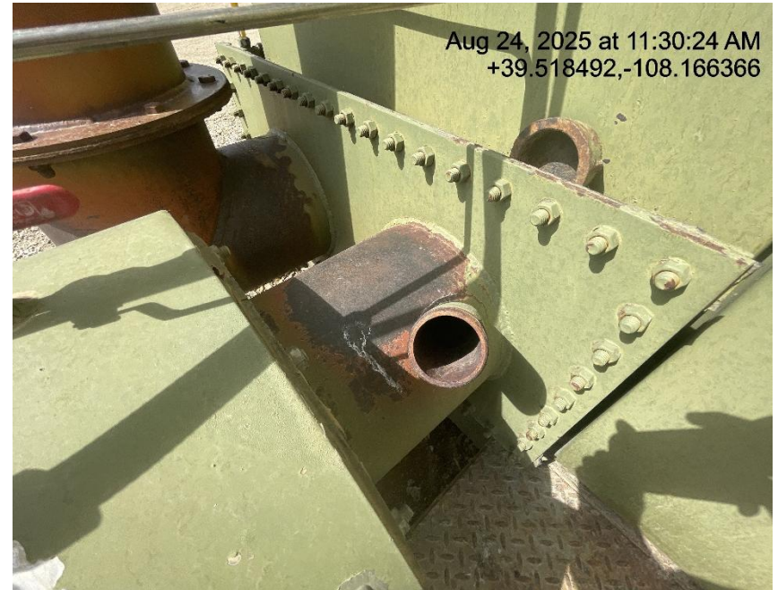
Photo # 2785 Open ended piping on fire tube/wildlife hazard
