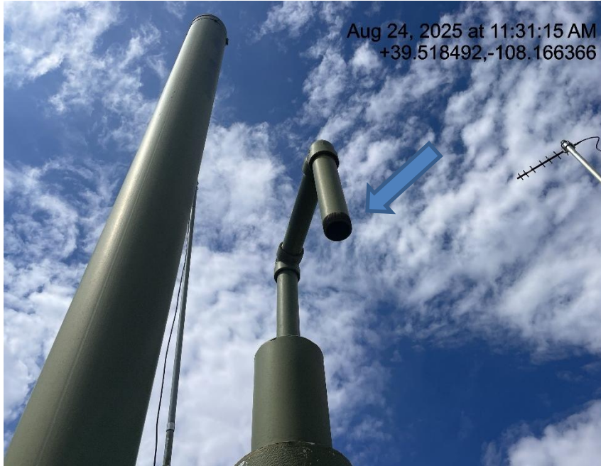
Photo # 2788 Open ended piping on dehy/wildlife hazard
