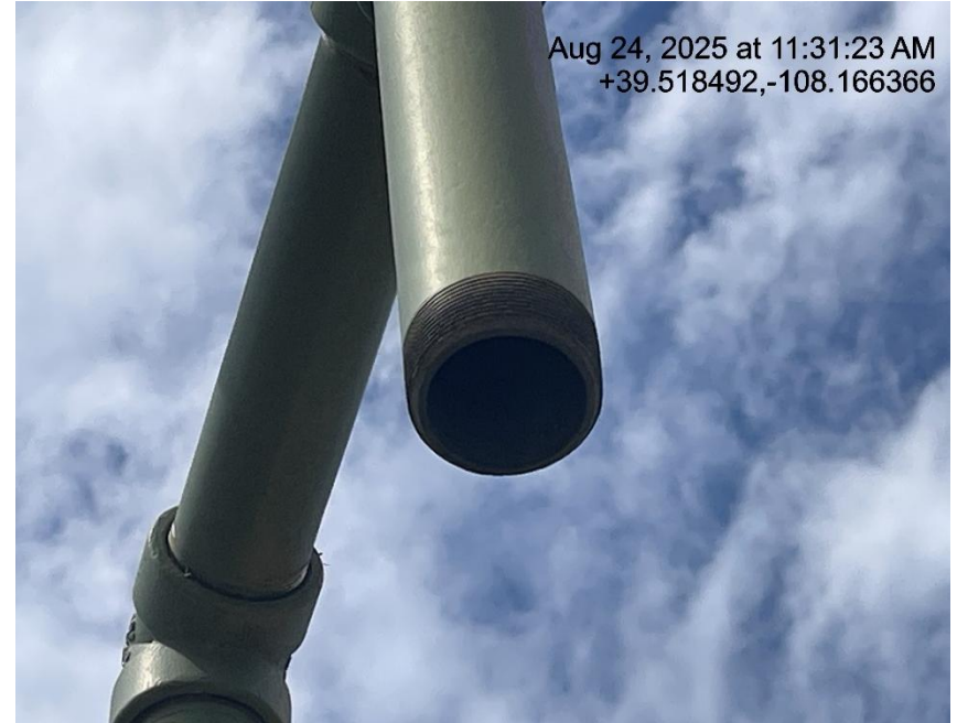
Photo # 2789 Open ended piping on dehy/wildlife hazard
