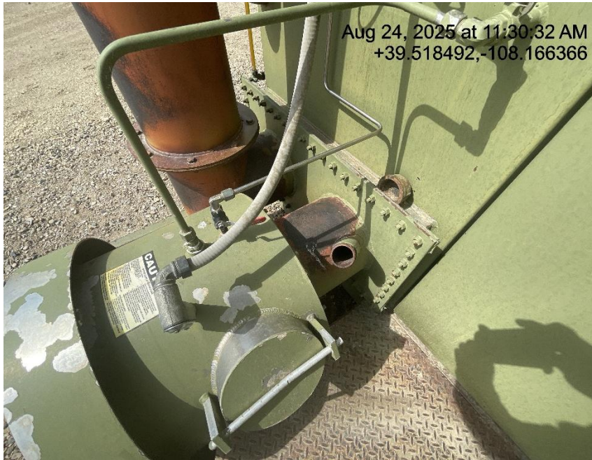
Photo # 2784 Open ended piping on fire tube/wildlife hazard
