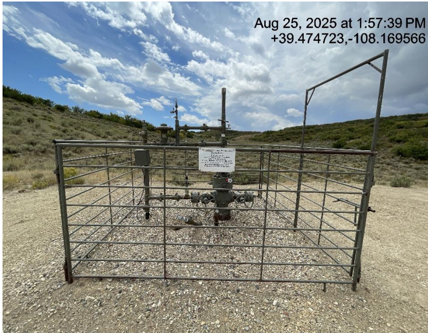
Photo # 4030 Wellhead sign has previous operators name
