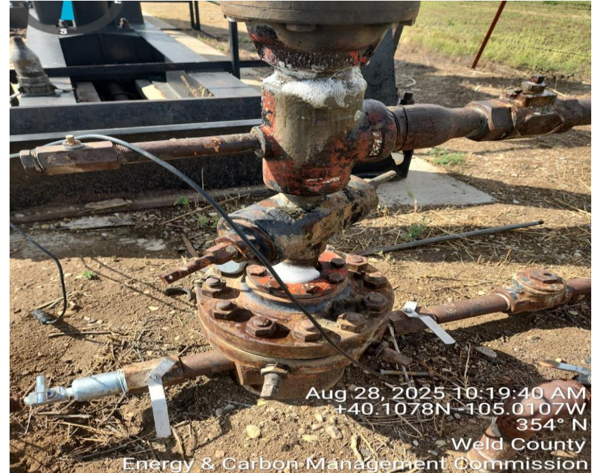
Soap test appears to be leaking
