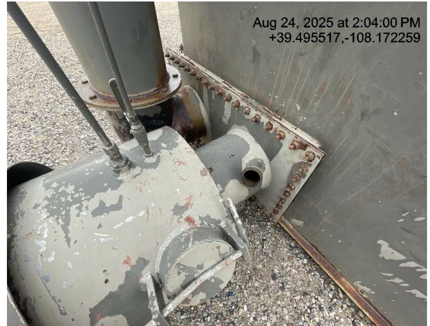
Photo # 3137 Open ended piping on fire tube/wildlife hazard
