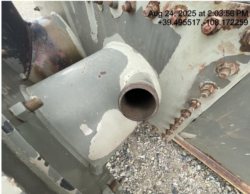
Photo # 3138 Open ended piping on fire tube/wildlife hazard
