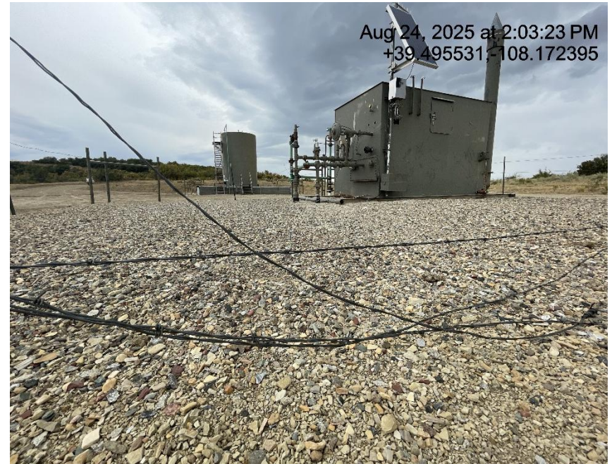
Photo # 3139 Barbed wire fence needs maintenance/wildlife & personnel hazard
