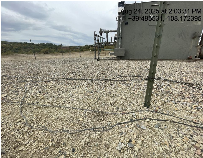
Photo # 3140 Barbed wire fence needs maintenance/wildlife & personnel hazard
