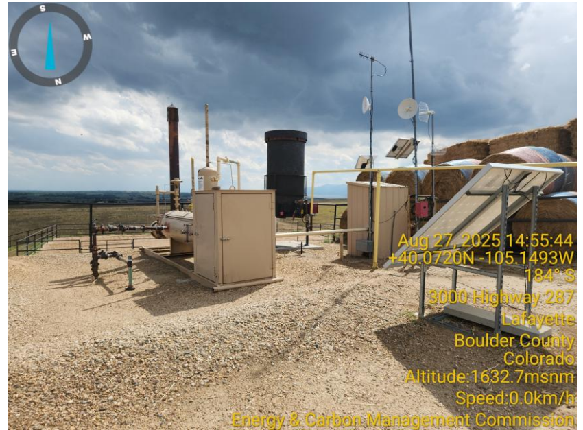
Photo 4 Horizontal Heated separator, gas meter run & ecd.
