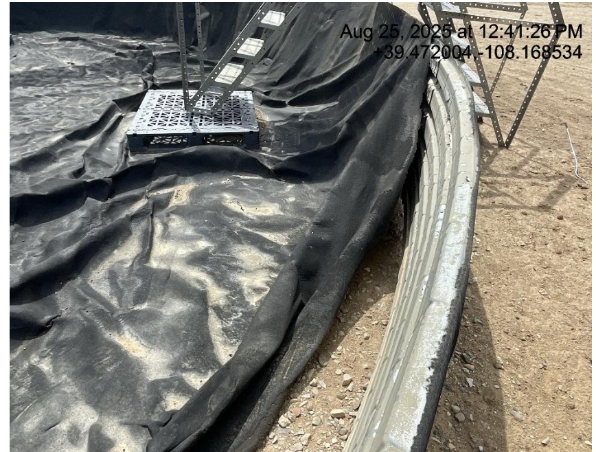
Photo # 3730 Secondary containment liner needs maintenance
