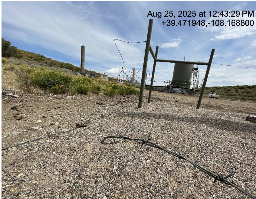
Photo # 3733 Barbed wire fence around separator needs maintenance/wildlife hazard
