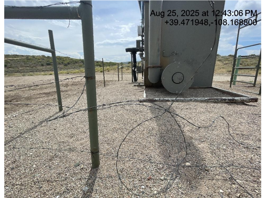
Photo # 3732 Barbed wire fence around separator needs maintenance/wildlife hazard
