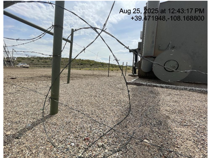
Photo # 3734 Barbed wire fence around separator needs maintenance/wildlife hazard
