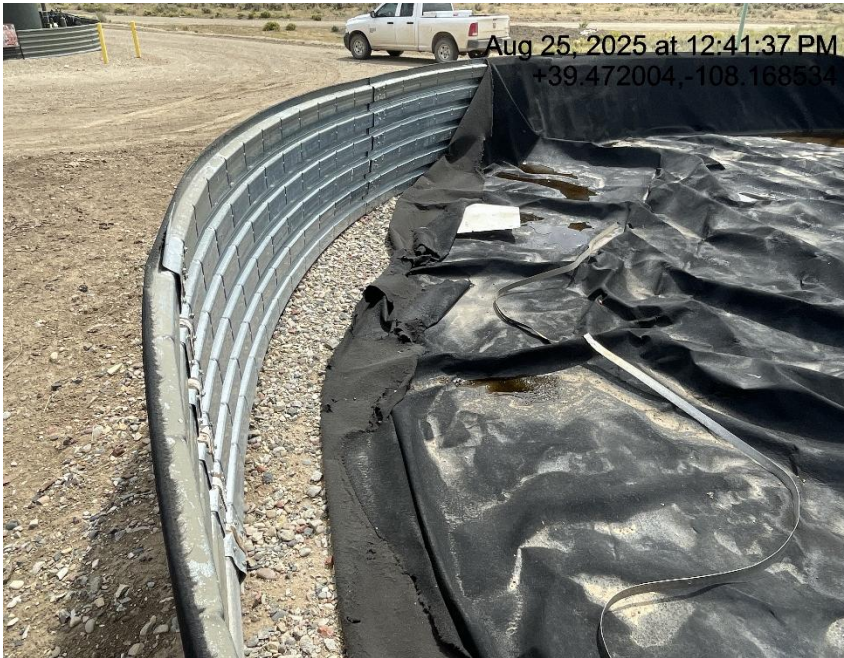
Photo # 3729 Secondary containment liner needs maintenance
