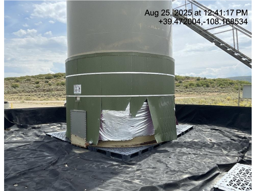
Photo # 3728 Tank lacks required labeling
