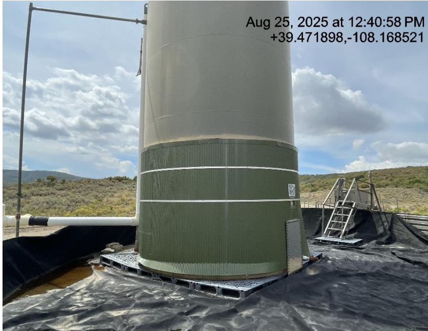
Photo # 3727 Tank lacks required labeling
