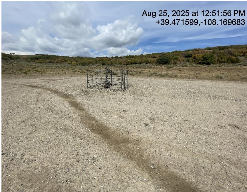
Photo # 3739 Stained soils
