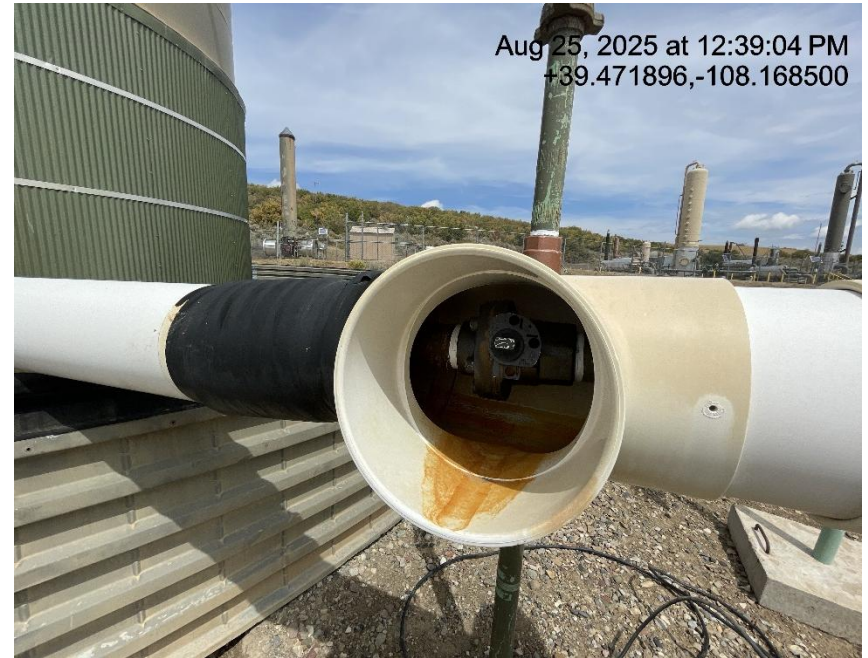
Photo # 3724 Flowline heating insulation open ended /wildlife hazard/available for entry by wildlife
