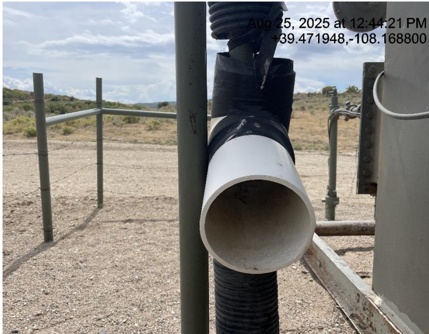
Photo # 3723 Flowline heating insulation open ended /wildlife hazard/available for entry by wildlife
