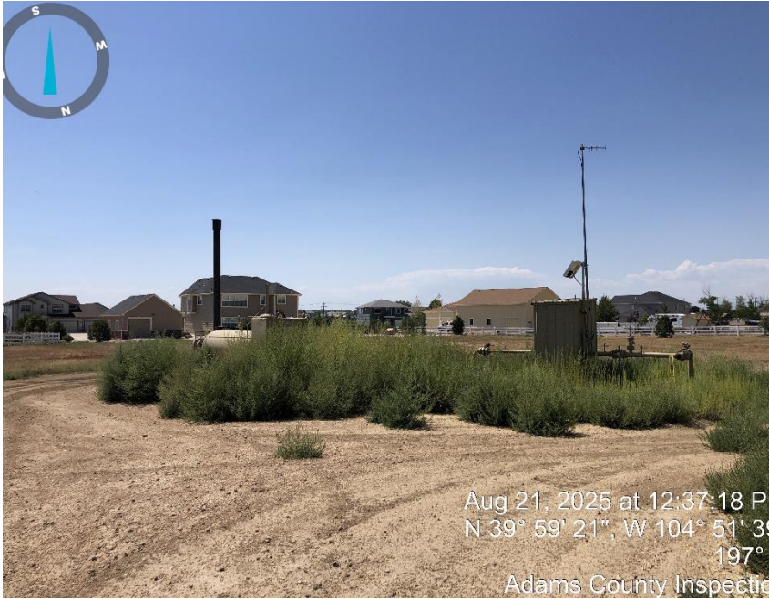
Photo #3 Separator, meter & weeds.
