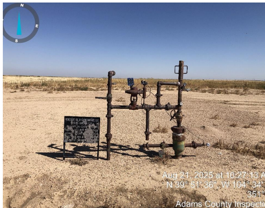
Photo #3 Well head.
