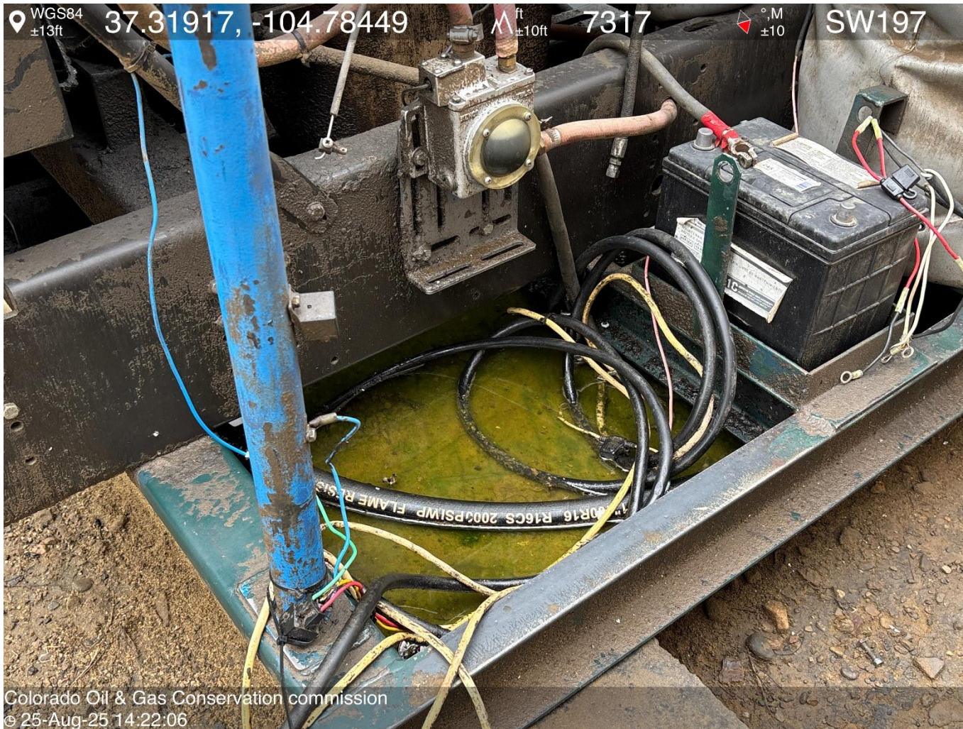
PHOTO 5: OILY WASTE AND APPEARS THERE MAY BE ANTIFREEZE IN PRIME MOVER SKID. DRAIN OILY WASTE REPAIR ALL LEAKS AND REMOVE IMPACTED SOIL PER RULE 1002..(2).D & 1002.f.(2)B, Comply with general provisions of the oil and gas act for wildlife protection AND SB-181, THIS IS THE SECOND NOTICE FOR THIS CA, IMMEDIATE ACTION IS REQUIRED.
