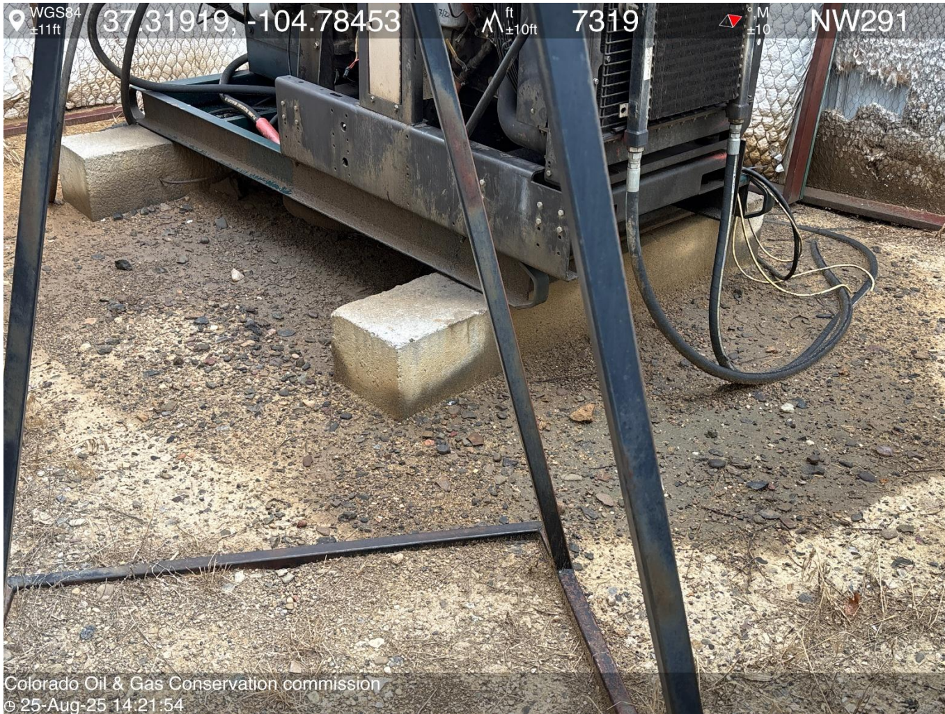
PHOTO 4: AREA OF IMPACTED SOIL AROUND PRIME MOVER SKID. Conduct maintenance on equipment, cleanup stained material and review self inspection processes. COMPLY WITH RULE 1002,(2).D, THIS IS THE SECOND NOTICE FOR THIS CA, IMMEDIATE ACTION IS REQUIRED.
