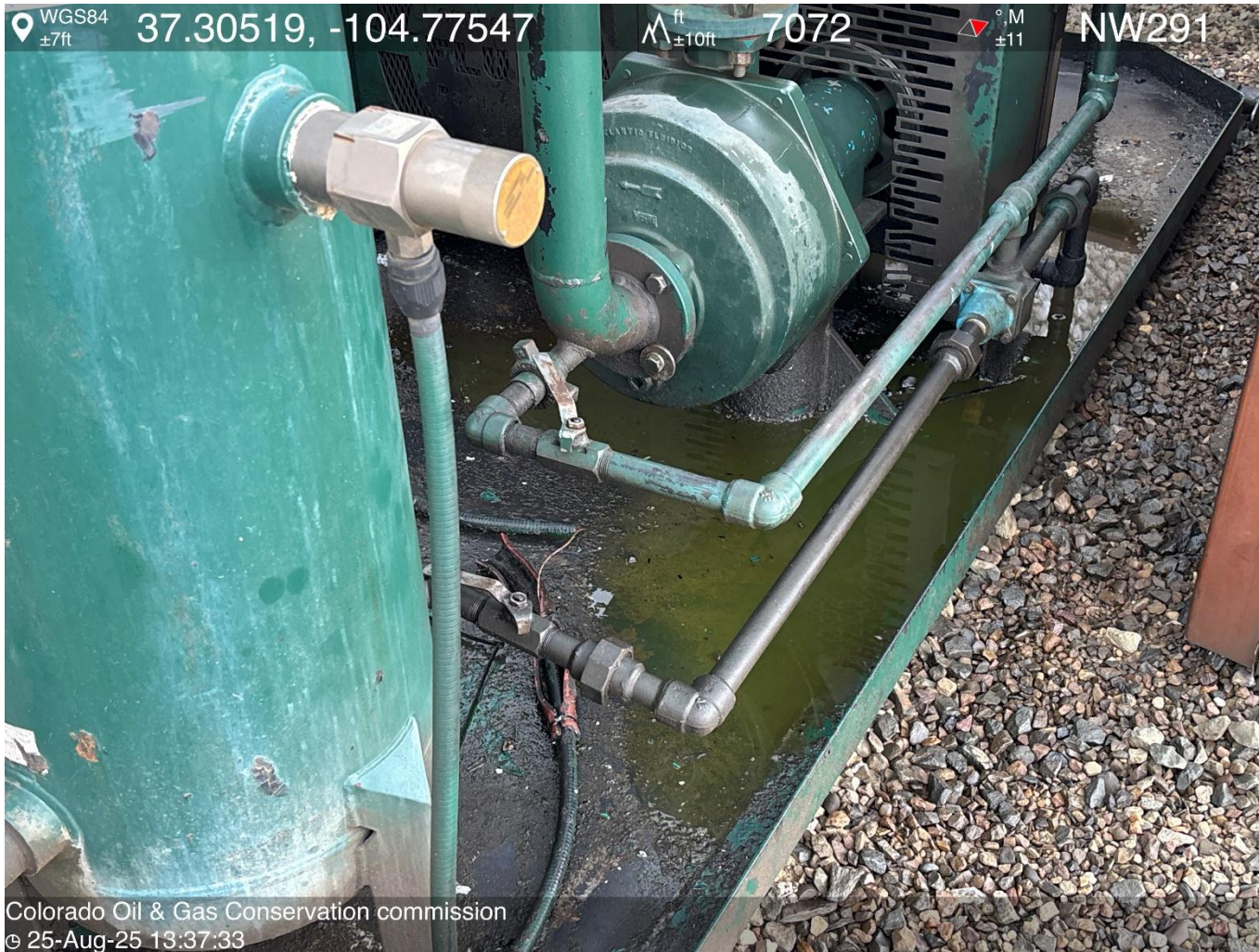
PHOTO 9: APPEARS TO BE ANTIFREEZE AND OILY WASTE IN COMPRESSOR SKID. DRAIN OILY WASTE REPAIR ALL LEAKS AND REMOVE IMPACTED SOIL PER RULE 1002..(2).D & 1002.f.(2)B, Comply with general provisions of the oil and gas act for wildlife protection AND SB-181. THIS IS THE SECOND NOTICE FOR THIS CORRECTIVE ACTION, IMMEDIATE ACTION IS REQUIRED.
