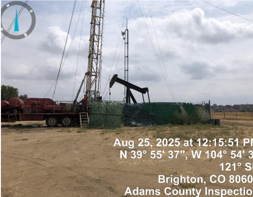
Photo#1 PUMPJACK/WORKOVER RIG ON WELL
