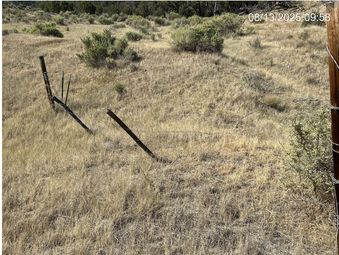
Photo 3: Photos shows an example of barbed-wire fencing surrounding the location that appears to be in disrepair. Comply with Rule 603.h.
