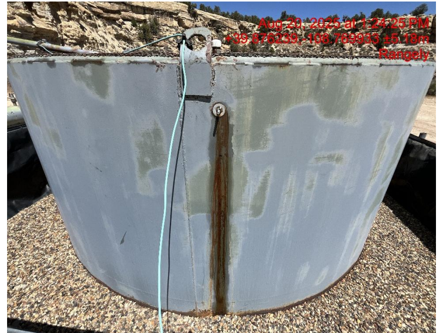
Photo # 2378 Possible leak on production tank/tank appears to lack integrity
