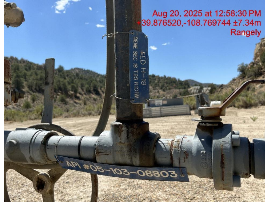
Photo # 2350 Wellhead sign lacks required information
