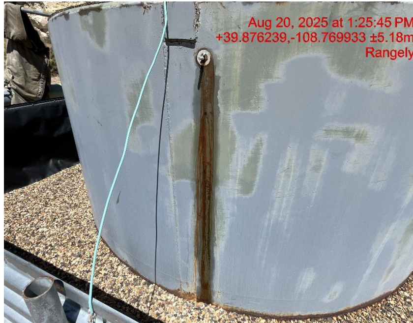
Photo # 2381 Possible leak on production tank/tank appears to lack integrity
