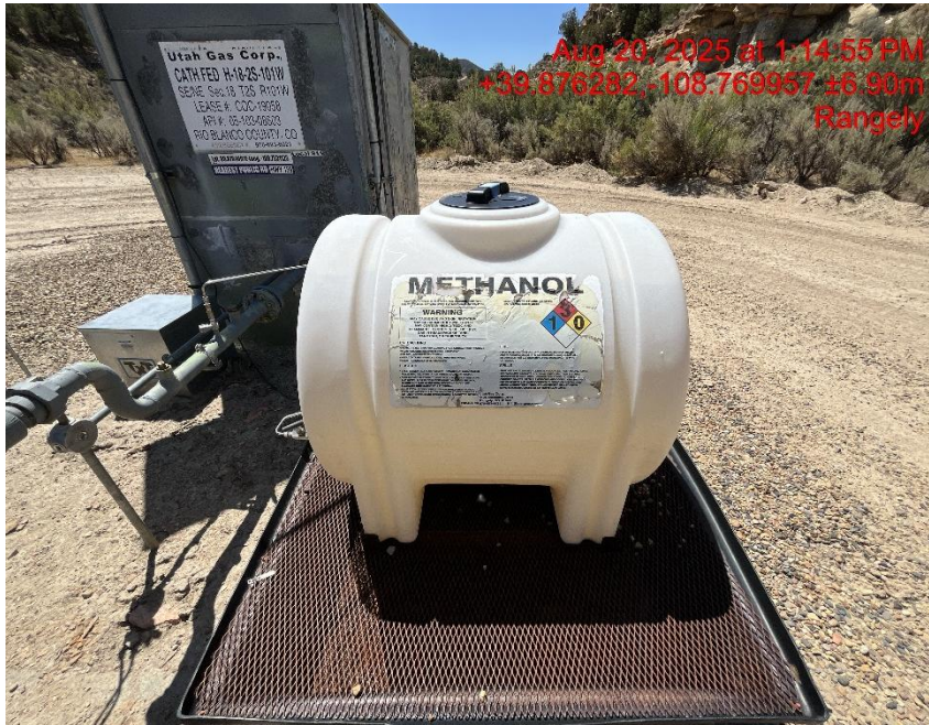
Photo # 2366 Chemical tank label is not legible/not in compliance with CECMC rules
