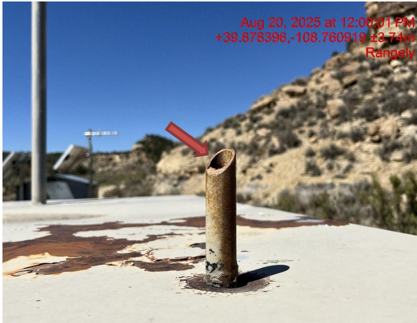
Photo # 2315 PRV vent line does not comply with CECMC pressure safety device rules
