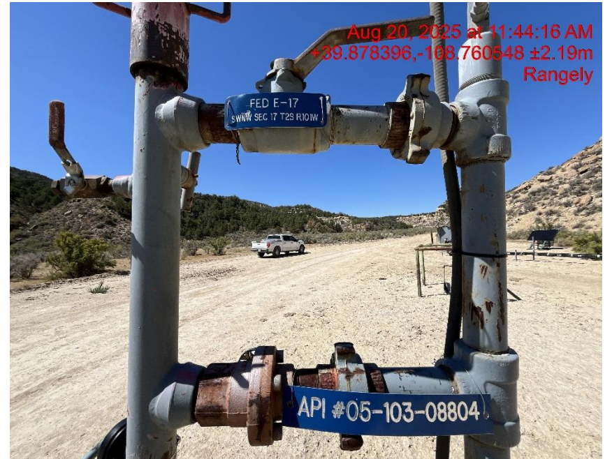
Photo # 2298 Wellhead sign lacks required information
