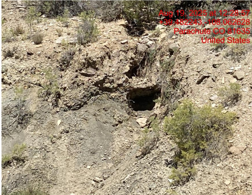
Insufficient Erosion Controls – Photo #00335
