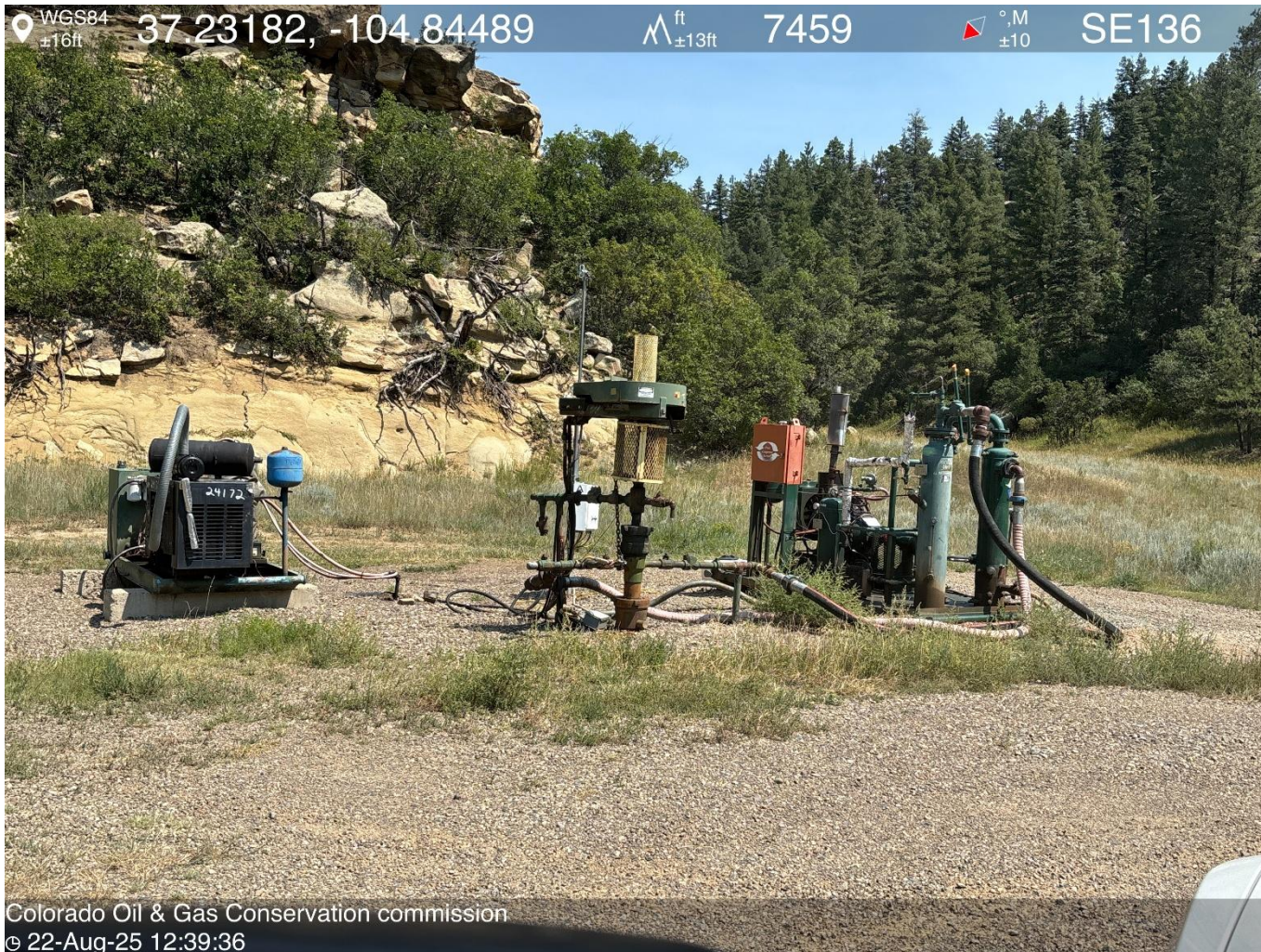
PHOTO 3: WELLHEAD AND EQUIPMENT.
