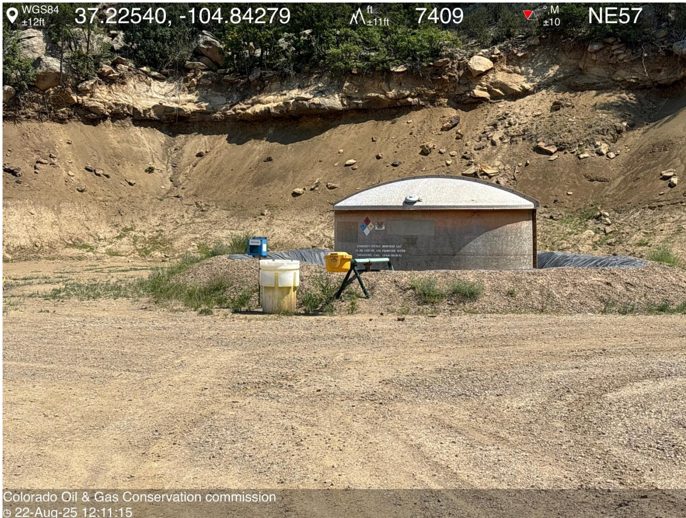
PHOTO 5: PRODUCED WATER TANK BATTERY.
