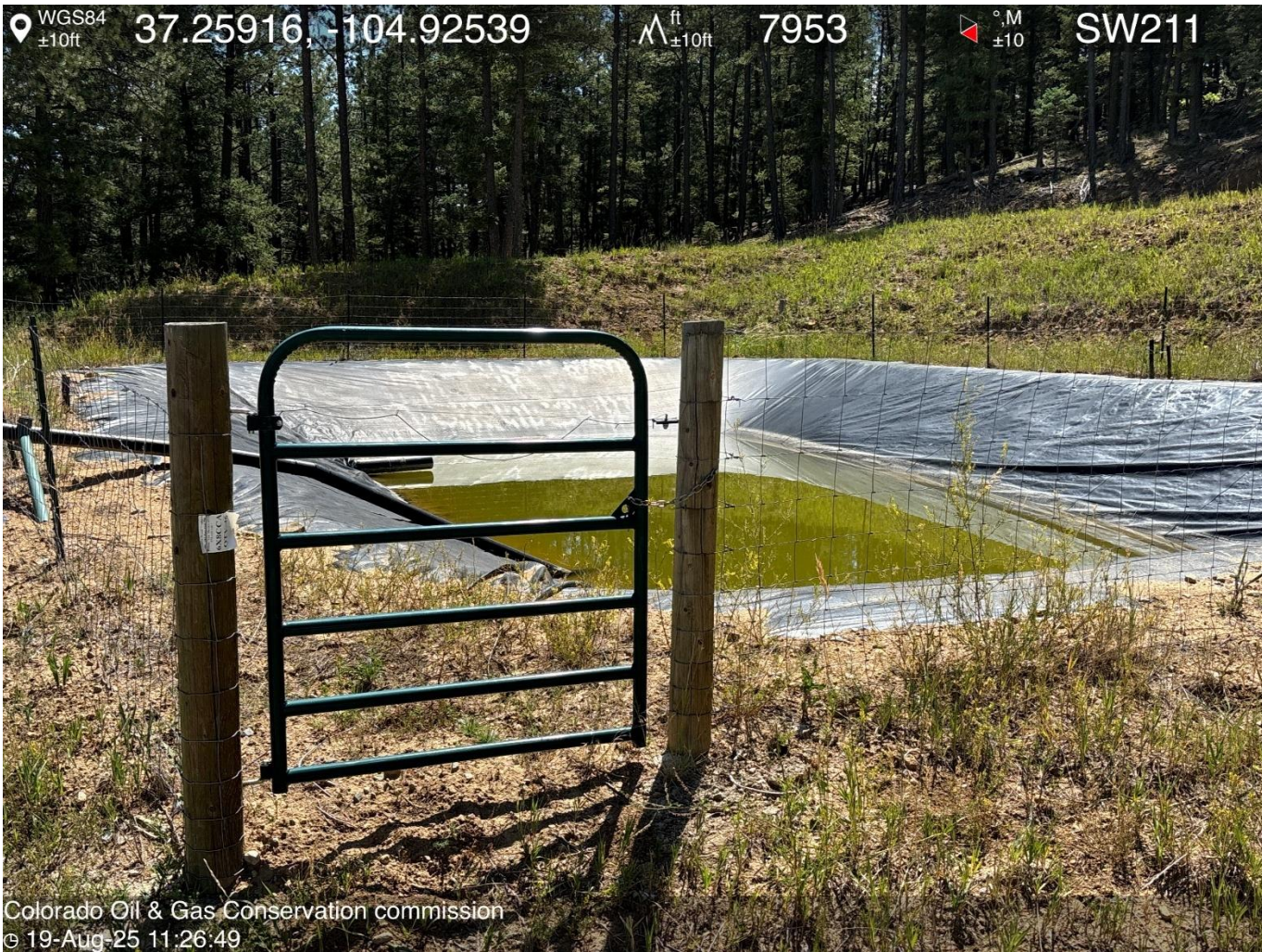
PHOTO 6: PRODUCED WATER EARTH PIT.
