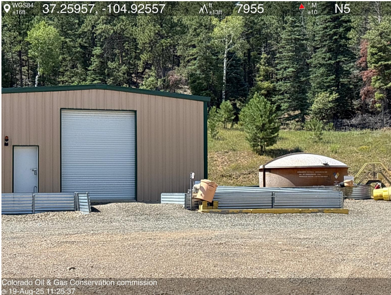
PHOTO 5: 210 BBL PRODUCED WATER TANK BATTERY AND FILTER HOUSE.
