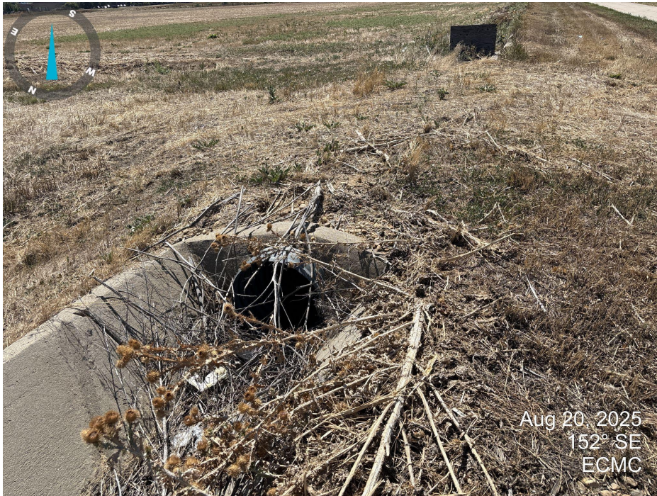
Photo 1. Picture taken at the center of the access road. Culvert is part of the irrigation system and appears to be used for landowner access to the field. List B noxious weed scotch thistle is present on the access road.
