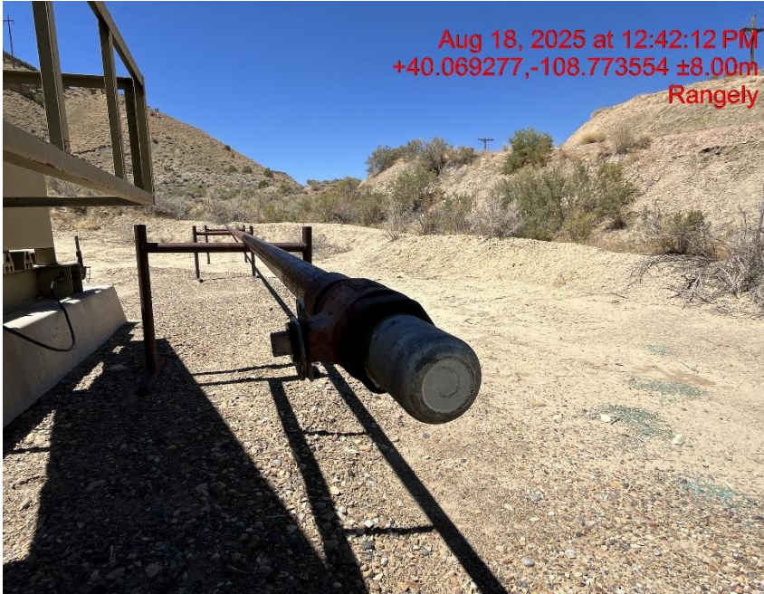
Photo # 2112 Unused flowline lacks lockout tagout (OOSLAT)
