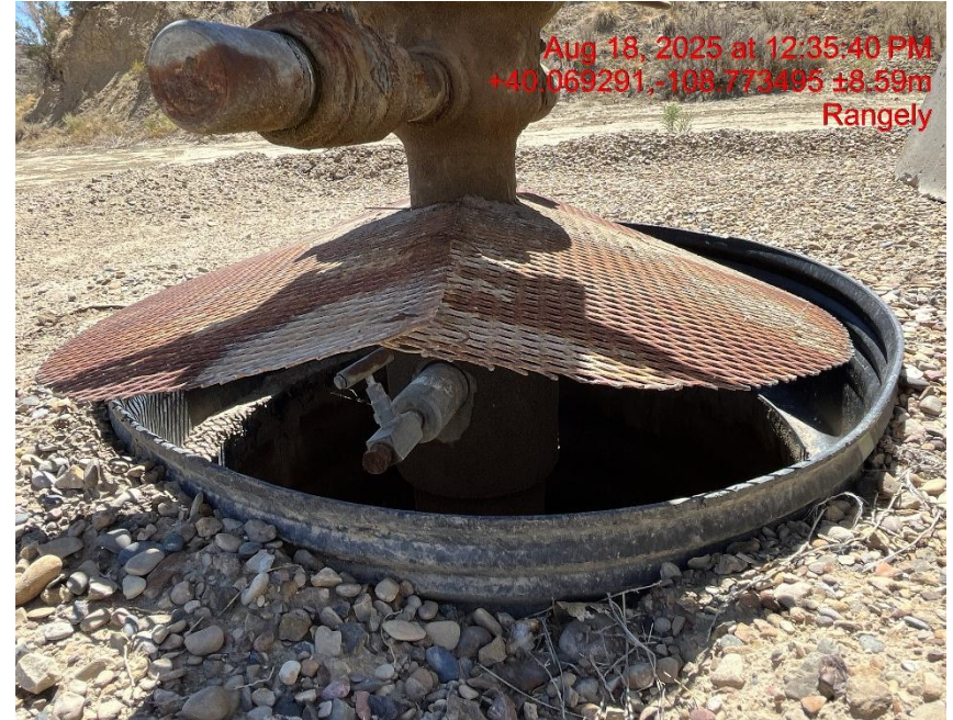
Photo # 2105 Improperly covered wellhead cellar lacks wildlife egress/available for entry by wildlife
