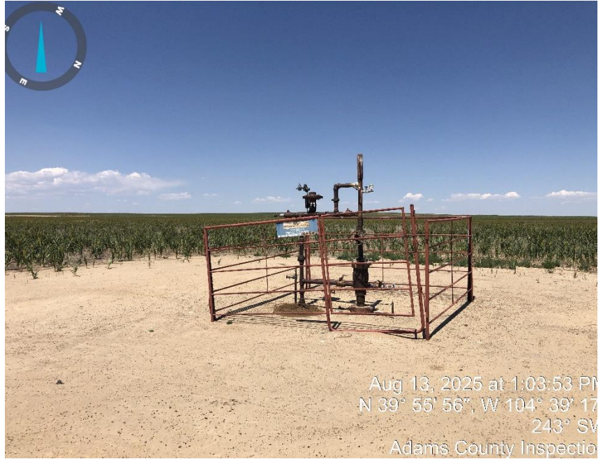
Photo #4 Well head.
