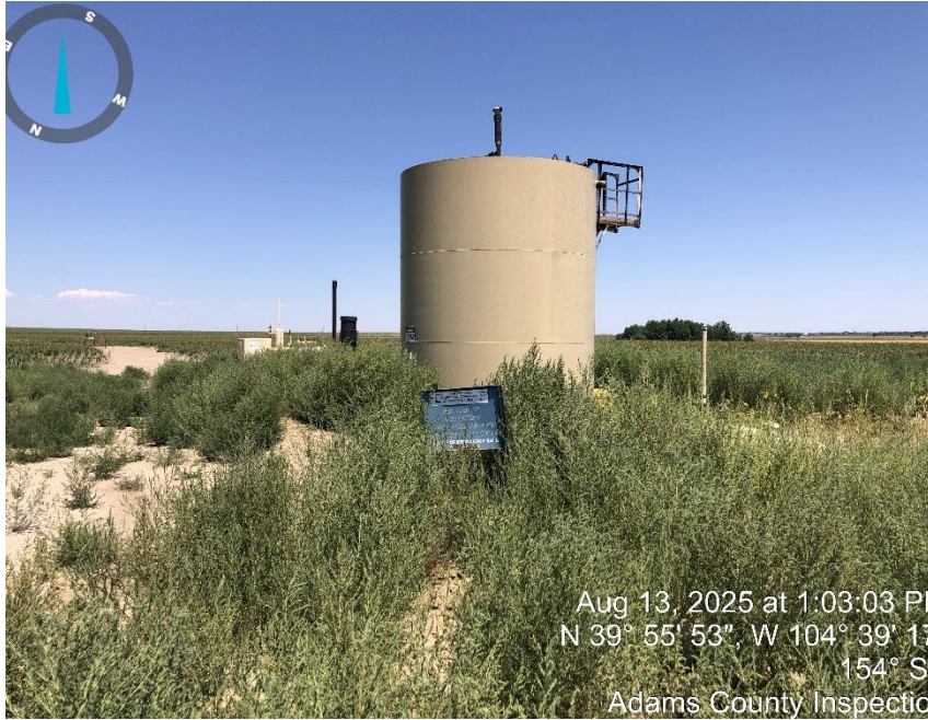
Photo #1 Tanks and weeds.
