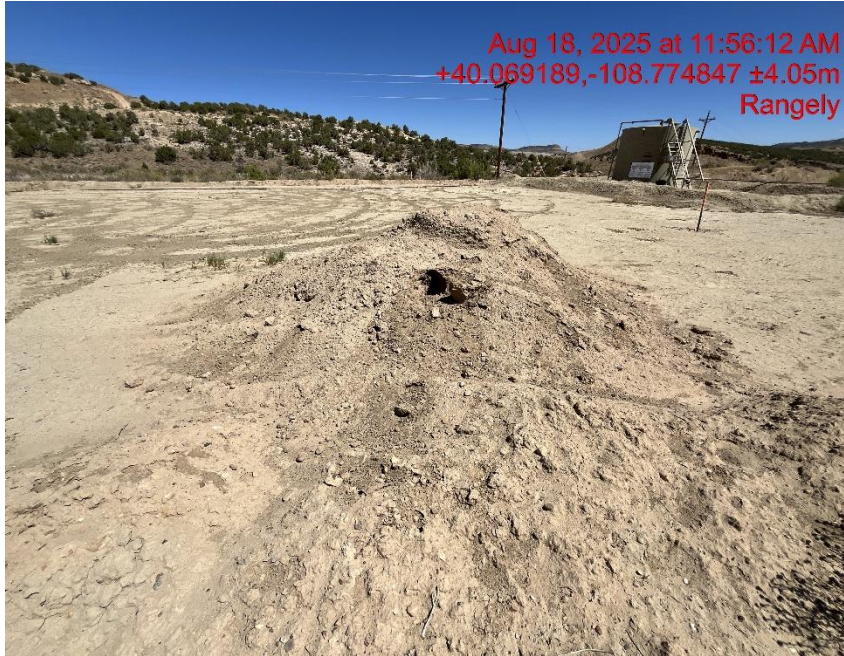
Photo # 2075 Stockpiled soils with no BMP's
