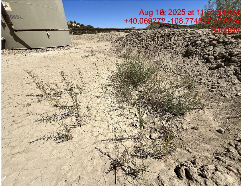
Photo # 2069 Small amount of weeds in secondary containment
