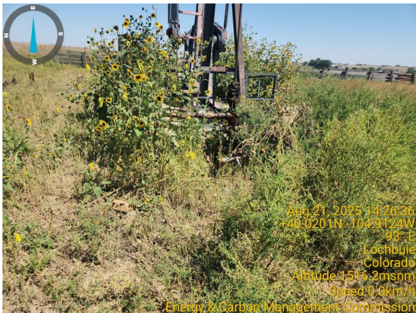
Photo 3 Tall vegetation around the wellhead.
