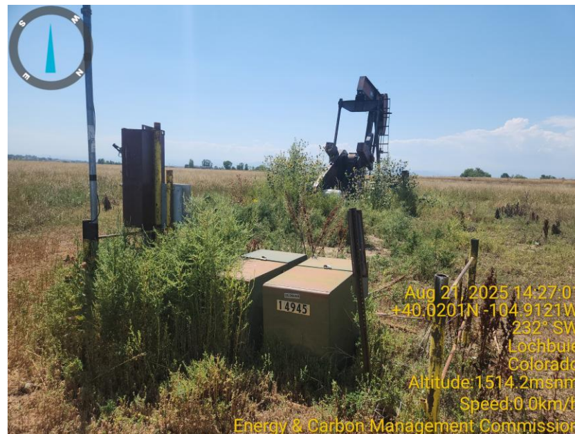
Photo 4 Ancillary equipment overrun with tall vegetation.
