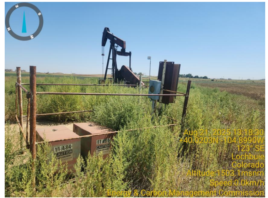
Photo 24 Ancillary equipment overrun with tall vegetation.
