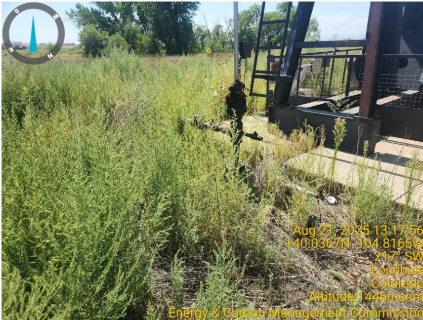
Photo 3 Tall vegetation around the wellhead.
