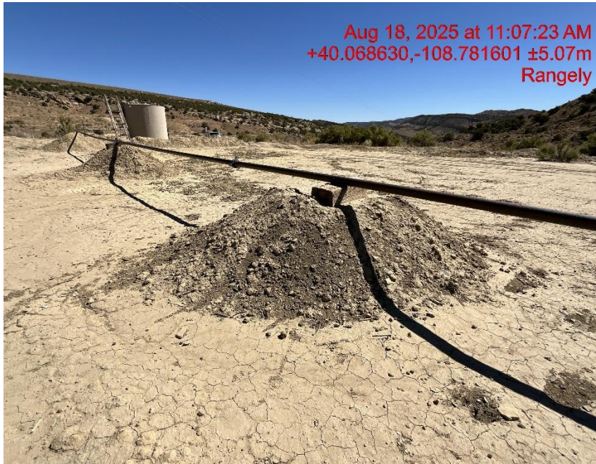
Photo # 2033 Stockpiled soils with no BMP's
