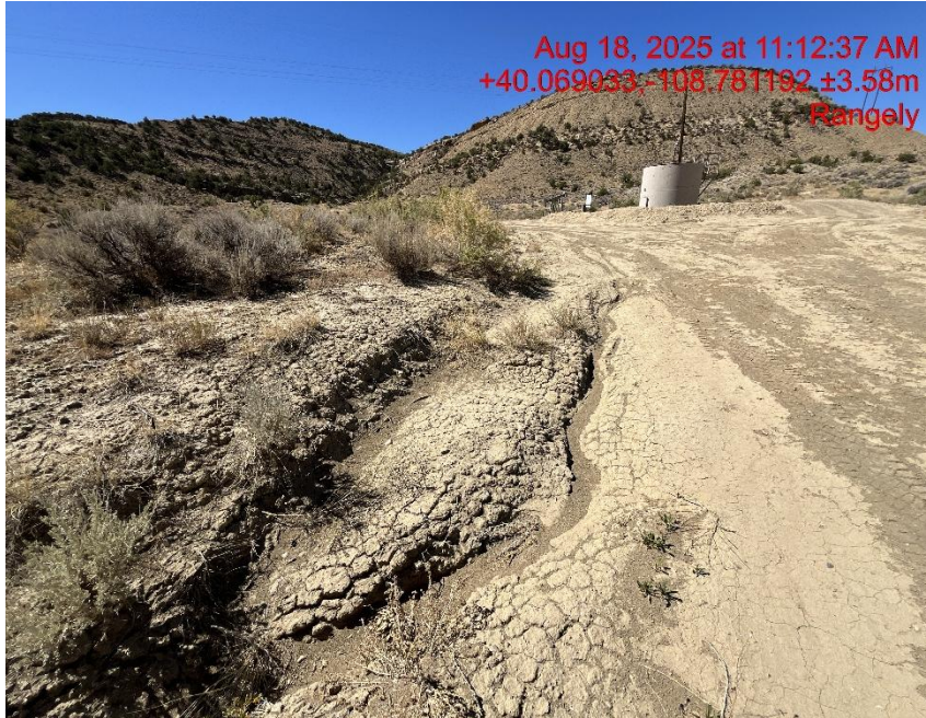
Photo # 2038 Failure to minimize erosion & transport of sediment off location/insufficient BMP's
