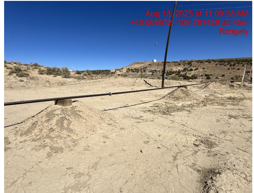
Photo # 2037 Stockpiled soils with no BMP's
