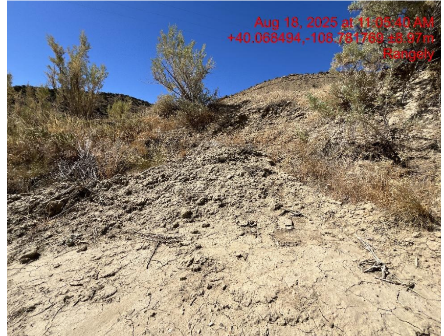
Photo # 2030 Stockpiled soils with no BMP's
