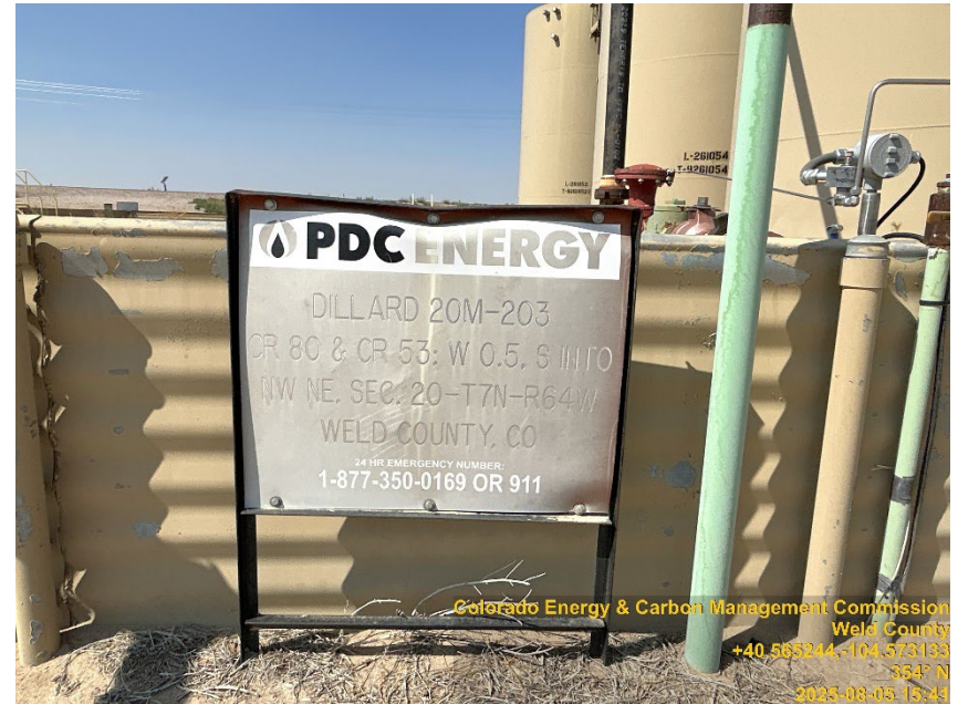
Photo #10 Dillard/20M-HZ Pad Battery site Active Battery / Facility signage #3
