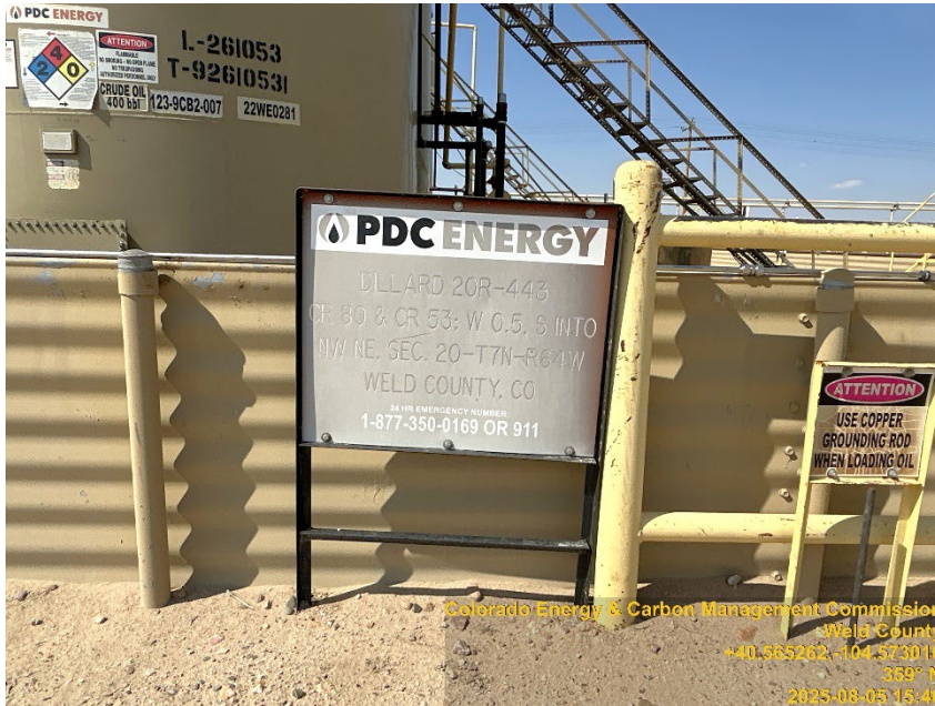
Photo #9 Dillard/20M-HZ Pad Battery site Active Battery / Facility signage #2
