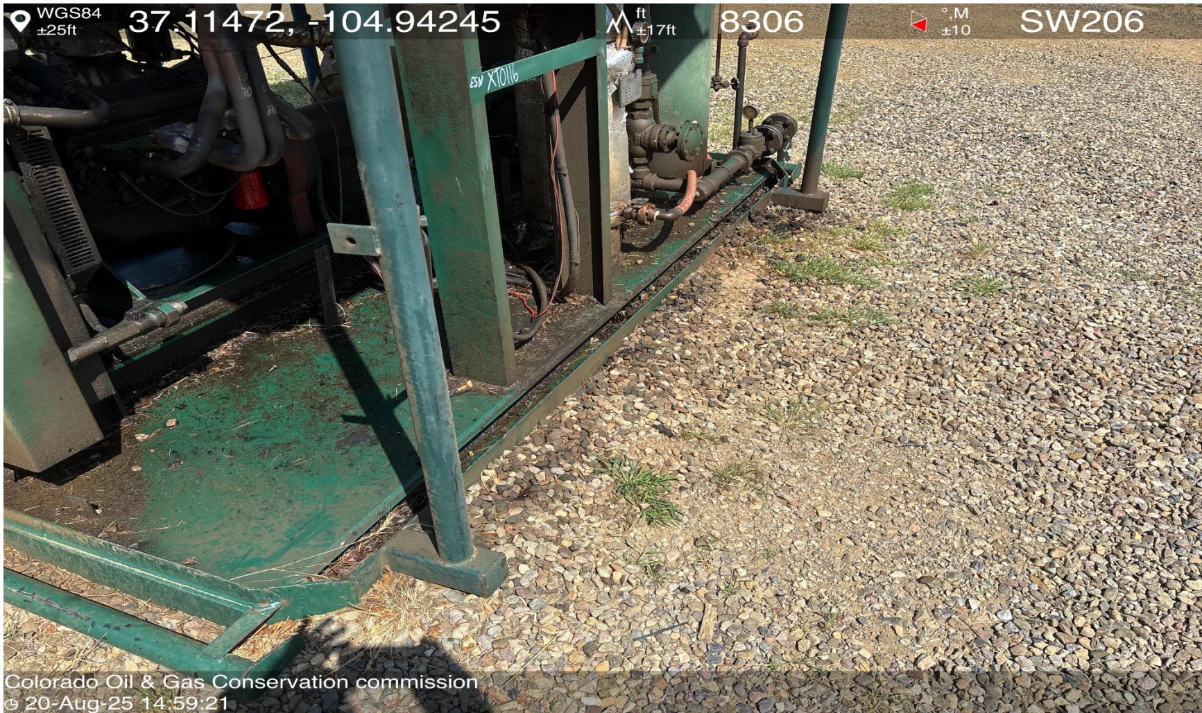
PHOTO 7: AREA OF IMPACTED SOIL NEAR COMPRESSOR SKID. Conduct maintenance on equipment, cleanup stained material and review self inspection processes. COMPLY WITH RULE 1002,.(2).D. THIS IS THE 2 ND NOTICE FOR THIS CA IMMEDIATE ACTION IS REQUIRED.
