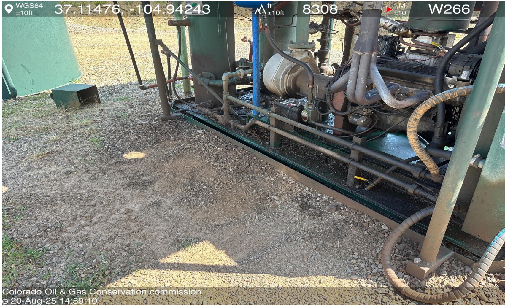
PHOTO 6: AREA OF IMPACTED SOIL NEAR COMPRESSOR SKID. Conduct maintenance on equipment, cleanup stained material and review self inspection processes. COMPLY WITH RULE 1002,(2).D. THIS IS THE 2 ND NOTICE FOR THIS CA IMMEDIATE ACTION IS REQUIRED.
