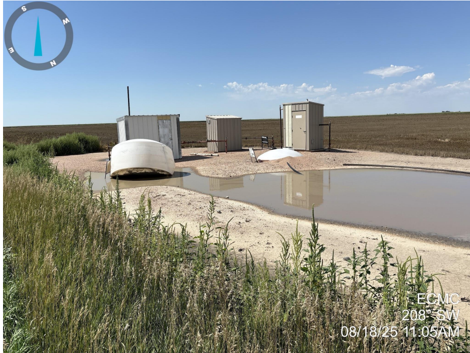
Photo 3. Photo taken of the tank battery location, facing southwest. See comments under Photo 1.
