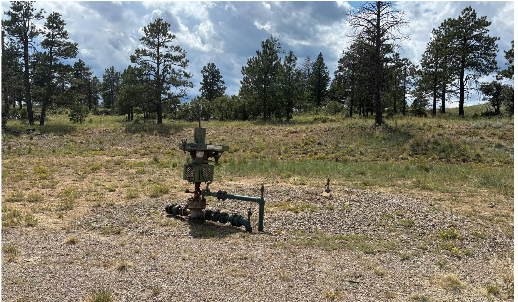
PHOTO 3: WELLHEAD AND EQUIPMENT.
