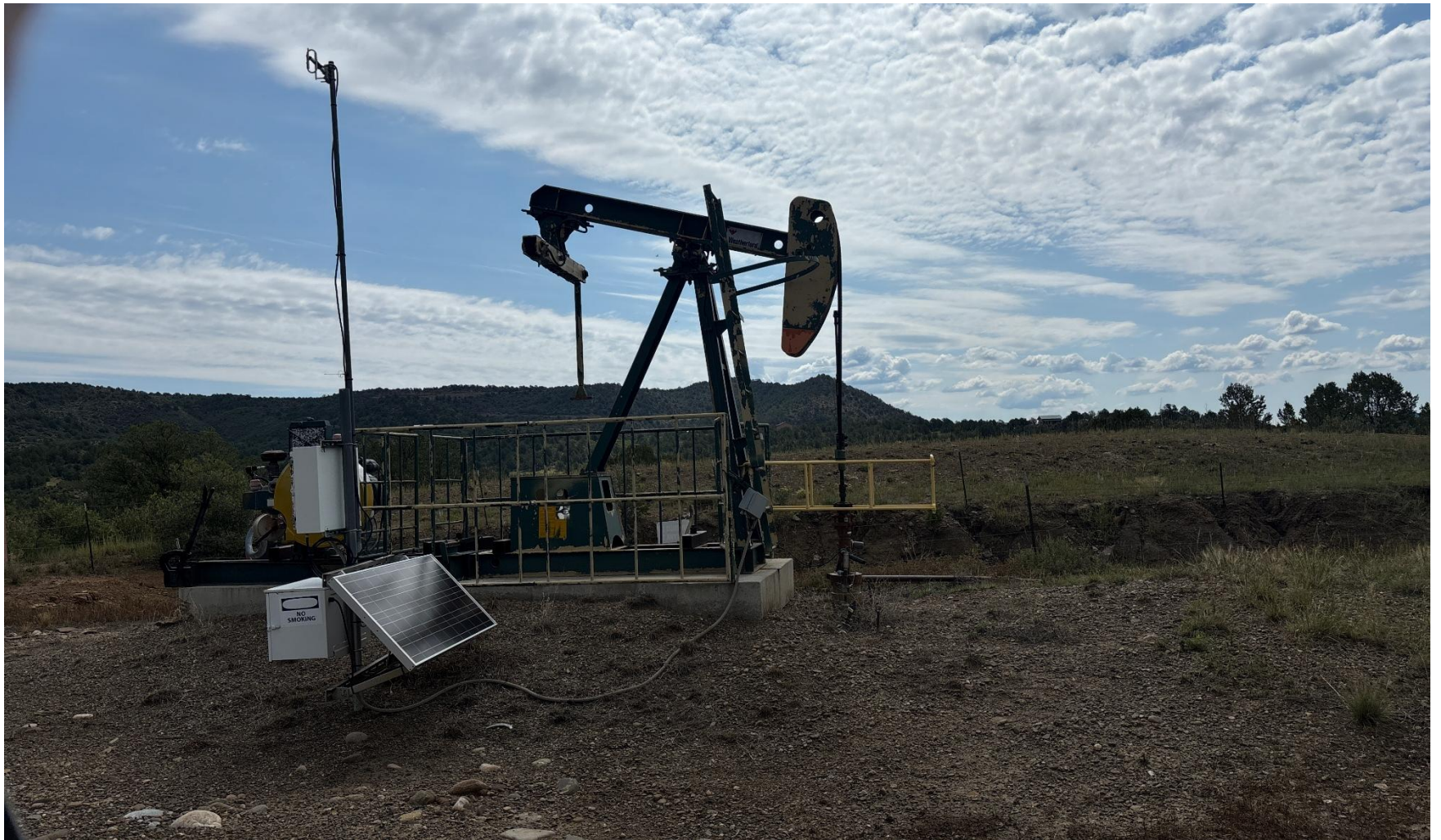
PHOTO 2: WELLHEAD AND EQUIPMENT.
