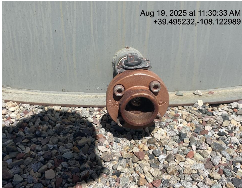
Photo # 1557 Open ended load line
