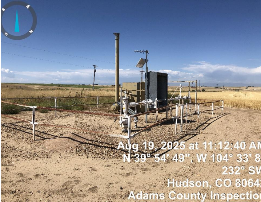
Photo#3 Separator/Gas Meter
