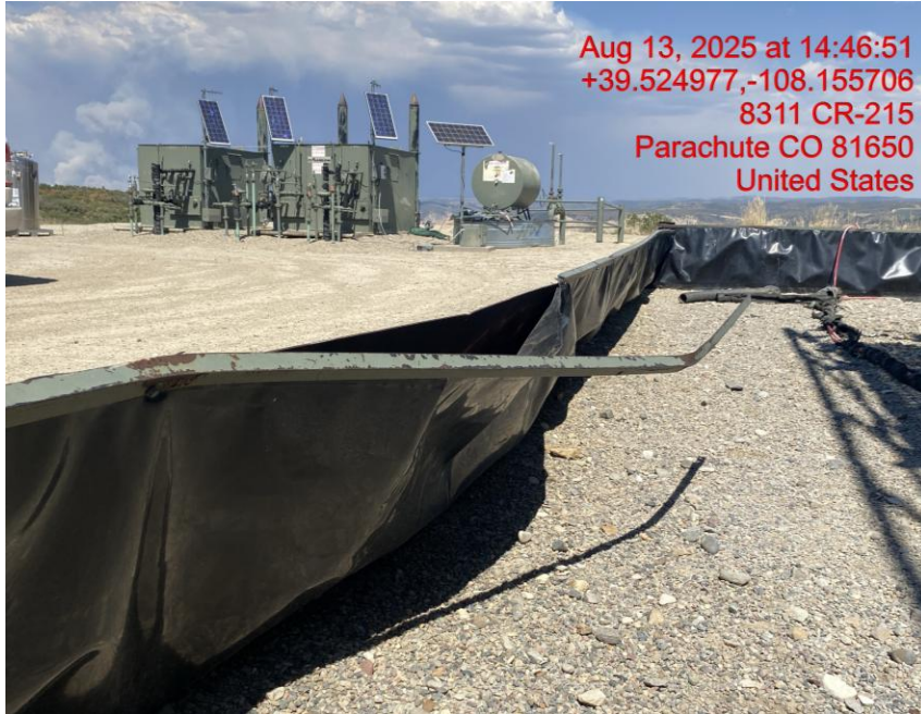
Damaged Berm – Photo #00196
