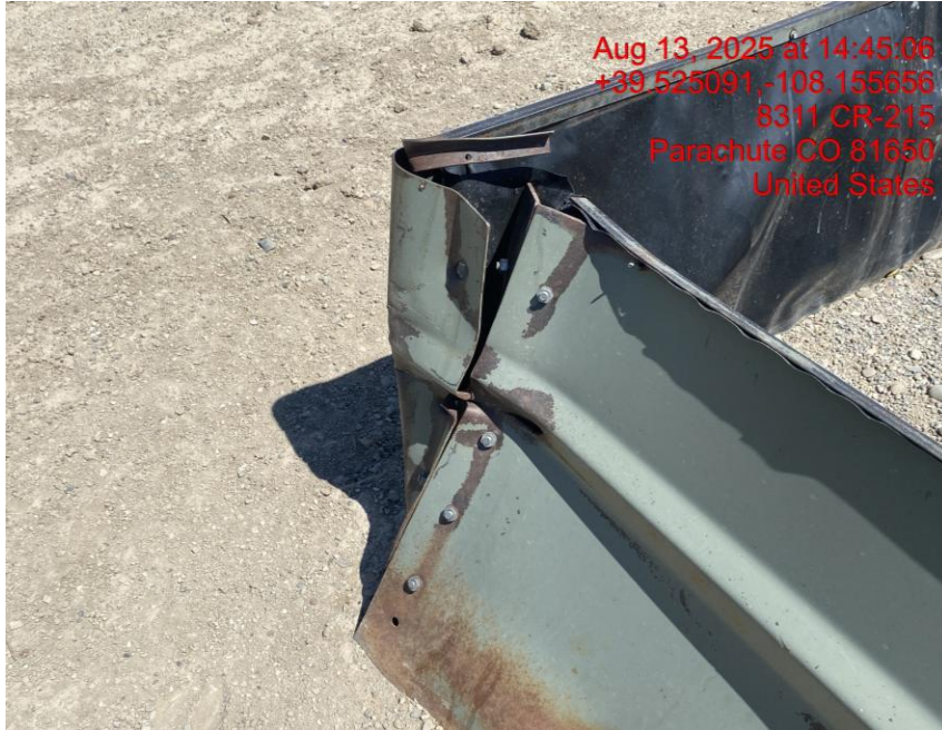
Damaged Berm – Photo #00189
